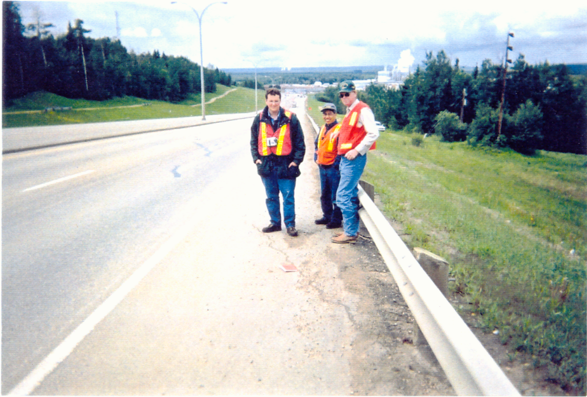
LOOKING WEST AT EAST CRACKS NEAR STATION 1+860
