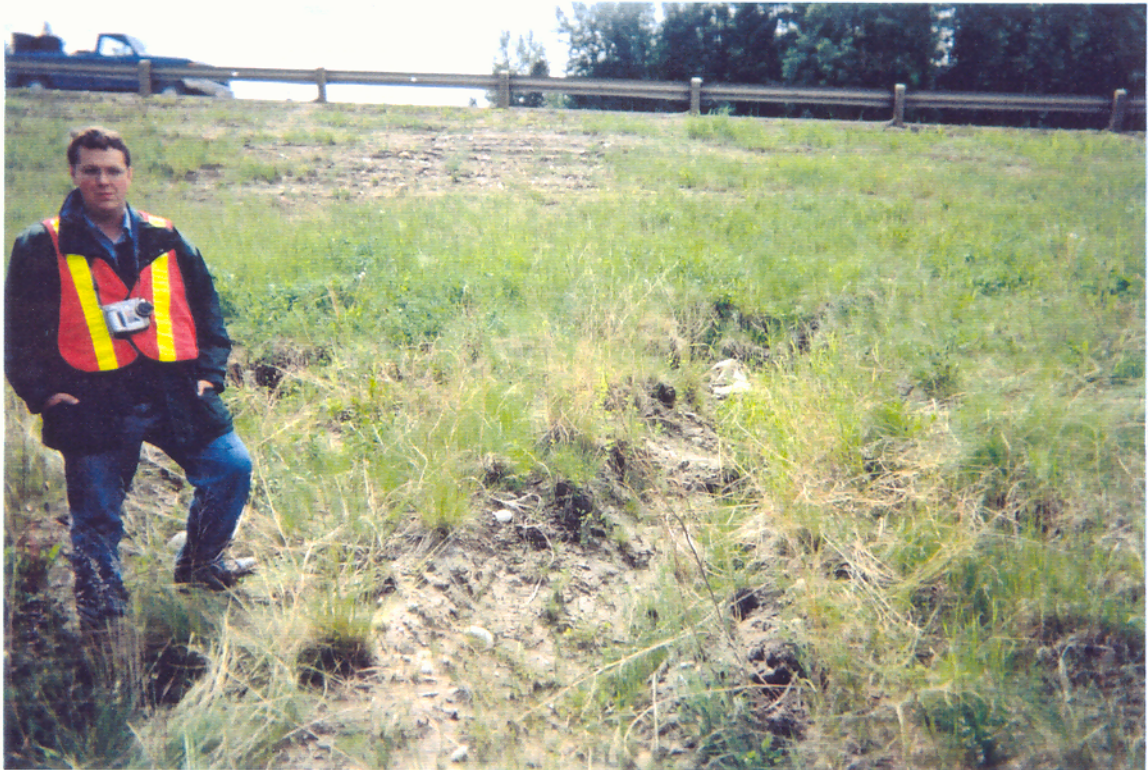
EROSION GULLIES NEAR STATION 1+920
