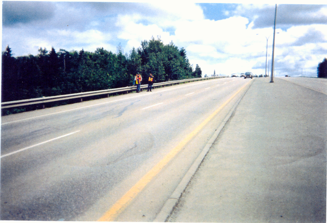
LOOKING NORTHEAST AT EAST CRACKS NEAR STATION 1+860
