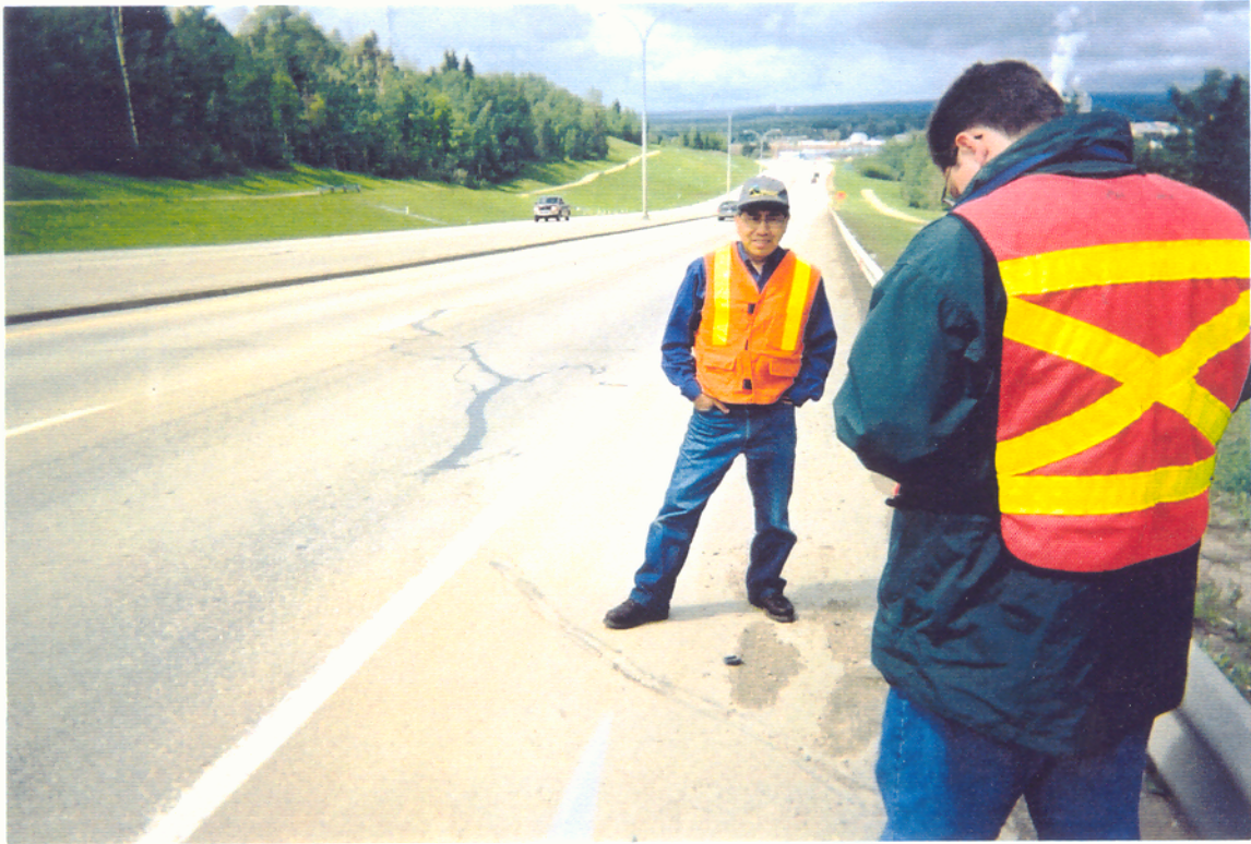
LOOKING WEST AT WEST CRACKS NEAR STATION 1+800
