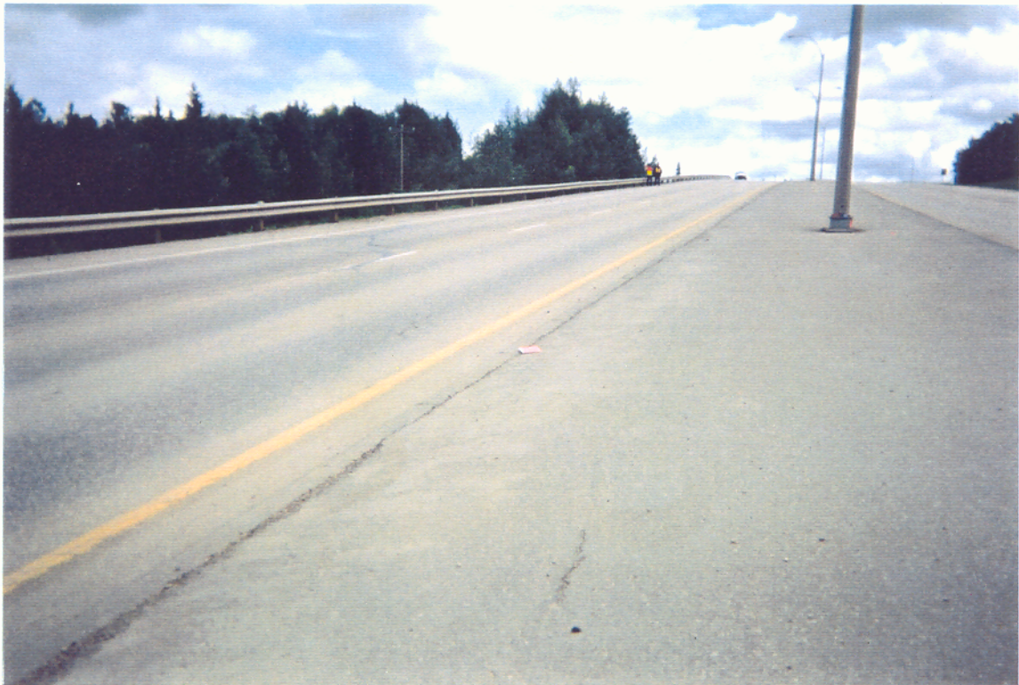
LOOKING NORTHEAST AT WEST CRACKS NEAR STATION 1+800
