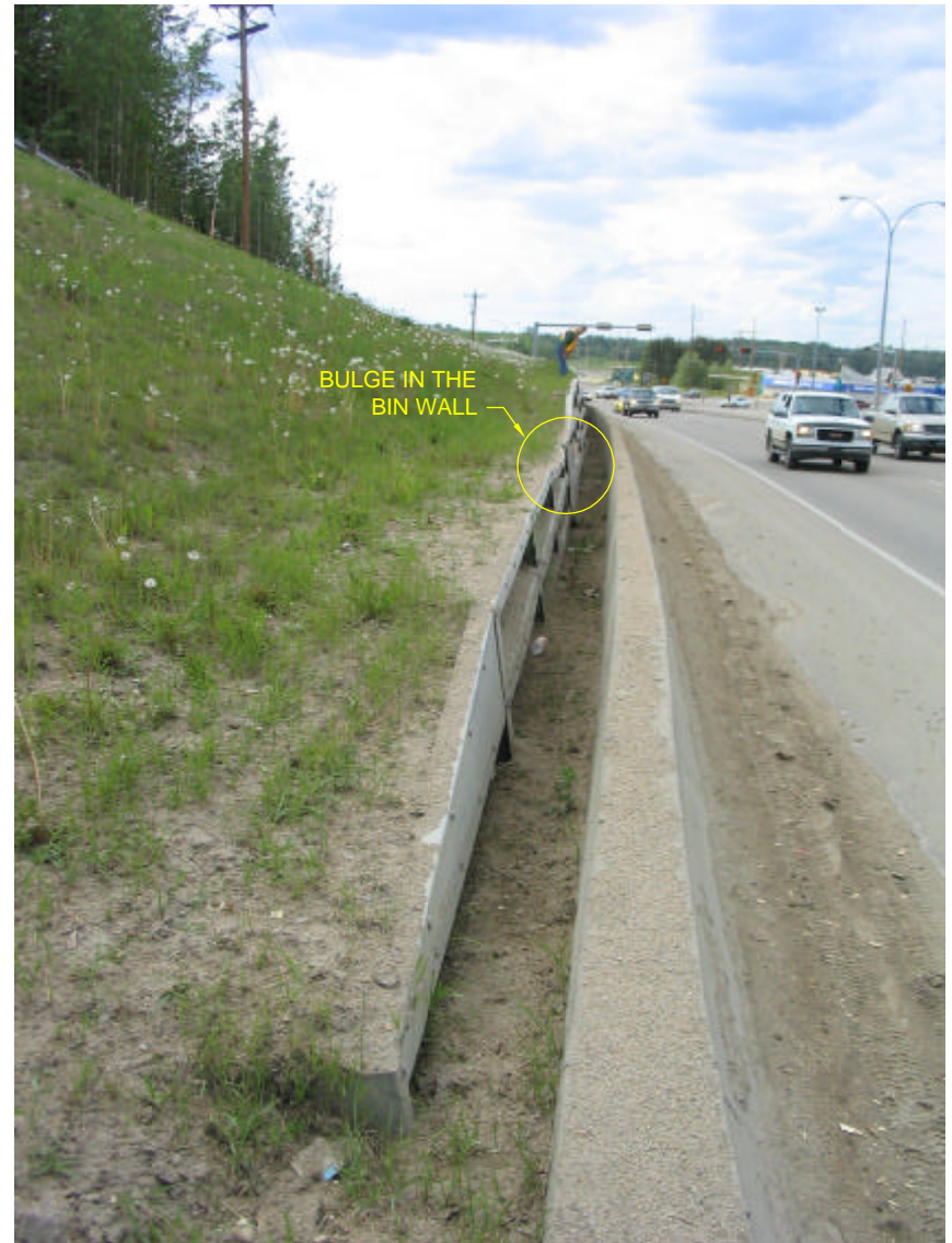
PHOTO 6 BULGE IN THE EAST SECTION OF THE BIN WALL
