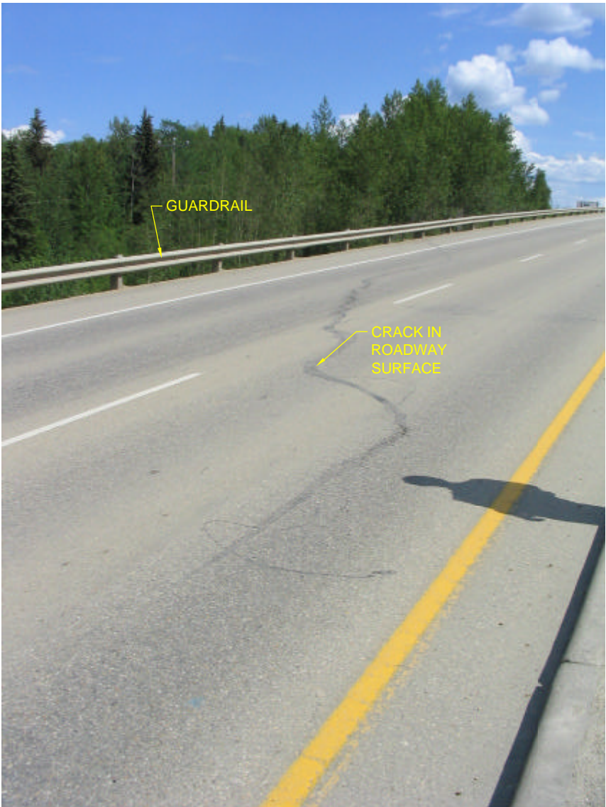
PHOTO 2 LOOKING EAST ON WESTBOUND LANES AT THE LOCATION OF ROADWAY EAST CRACK
