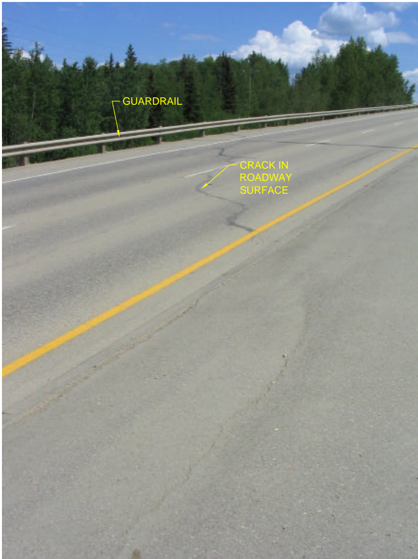
PHOTO 1 LOOKING EAST ON WESTBOUND LANES AT THE LOCATION OF ROADWAY WEST CRACK
