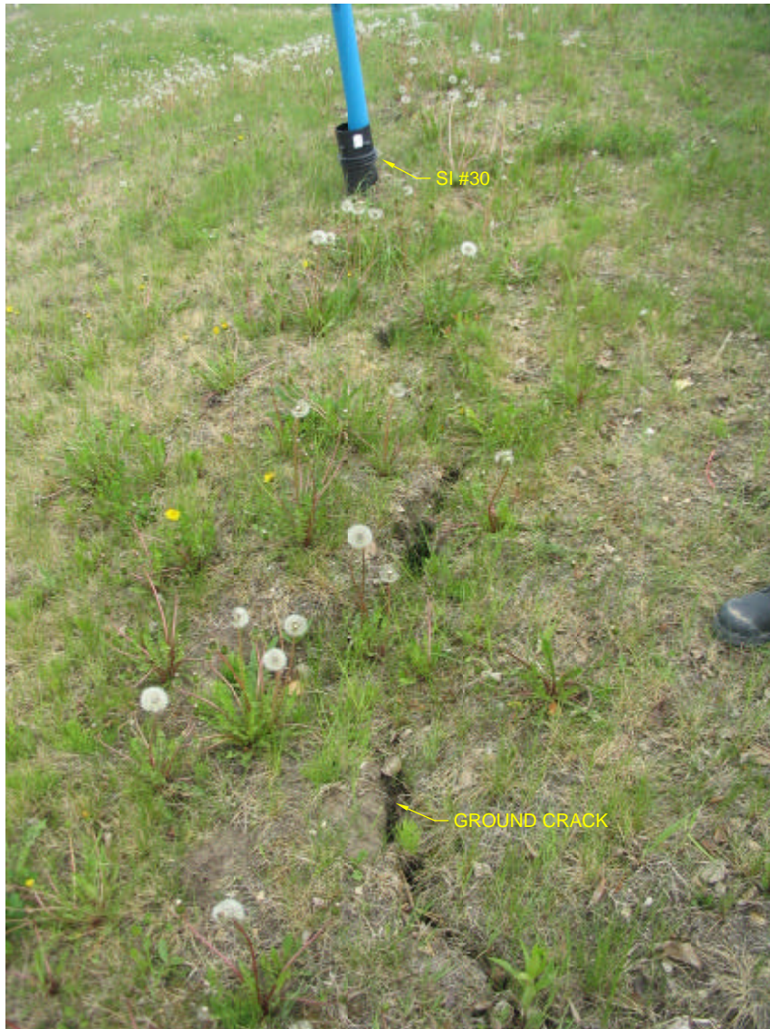
PHOTO 5 CRACK IN THE BACKSLOPE ABOVE THE BIN WALL
