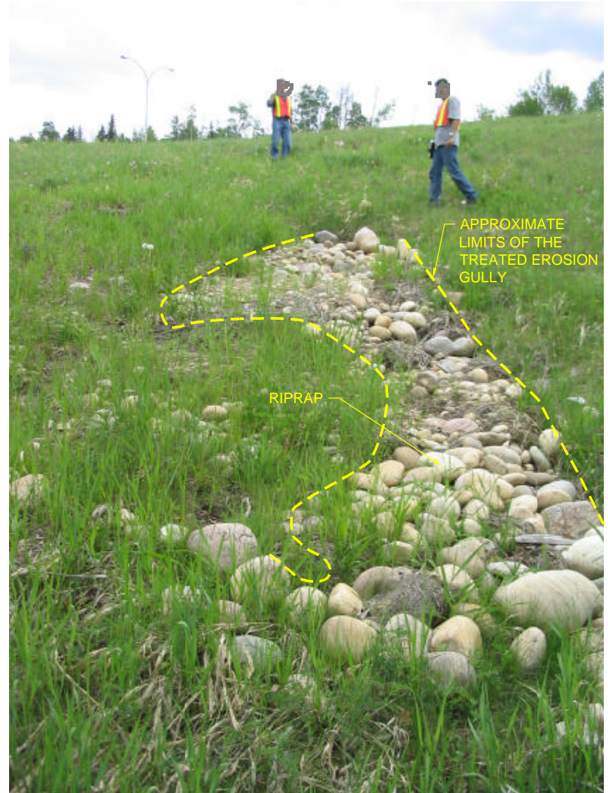
PHOTO 4 AN EROSION GULLY ON THE ROADWAY DOWNSLOPE TREATED WITH RIPRAP
