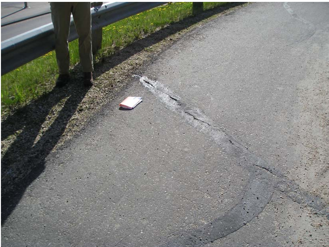
Photo 8 – Tension crack in paved trail southwest of bin wall. May 31, 2005
