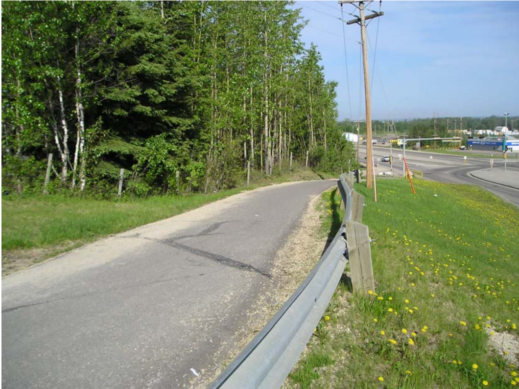
Photo 7 – Tension crack in paved trail southwest of bin wall (looking west).
