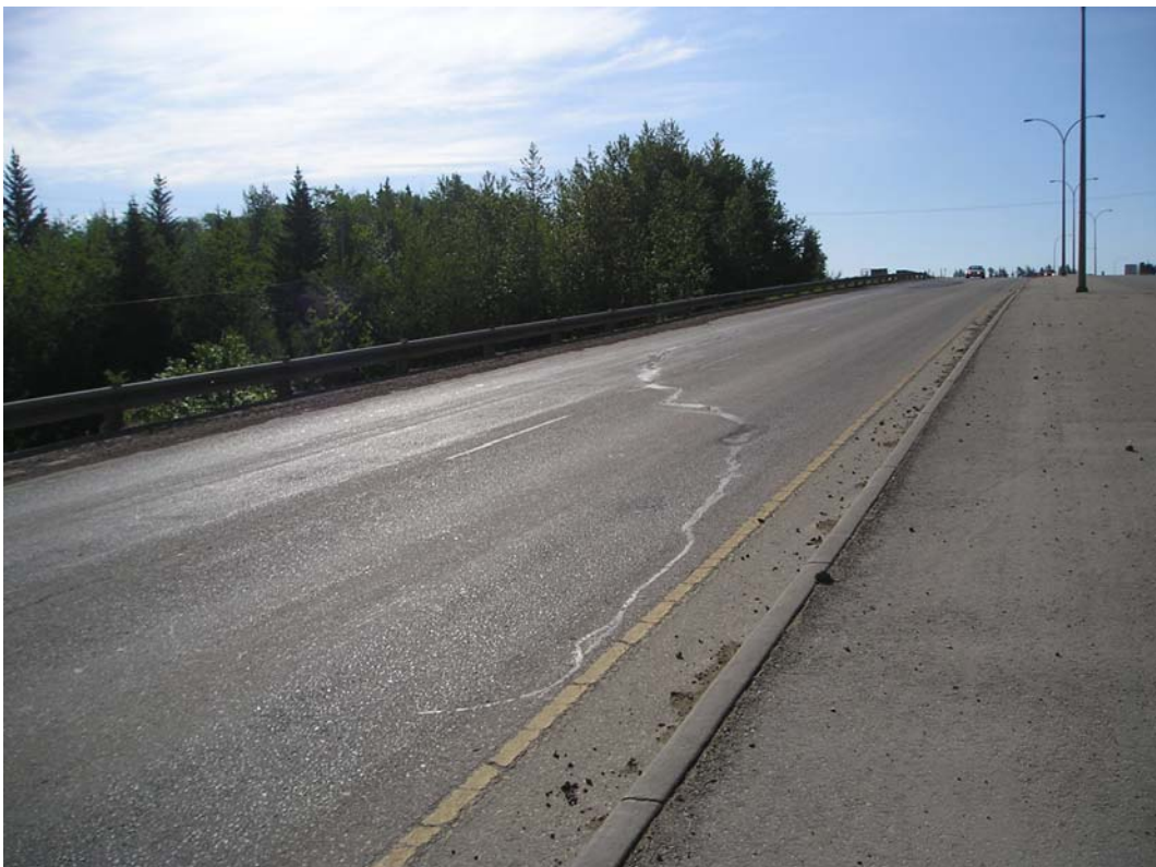
Photo 2 – Looking northeast at east crack.
