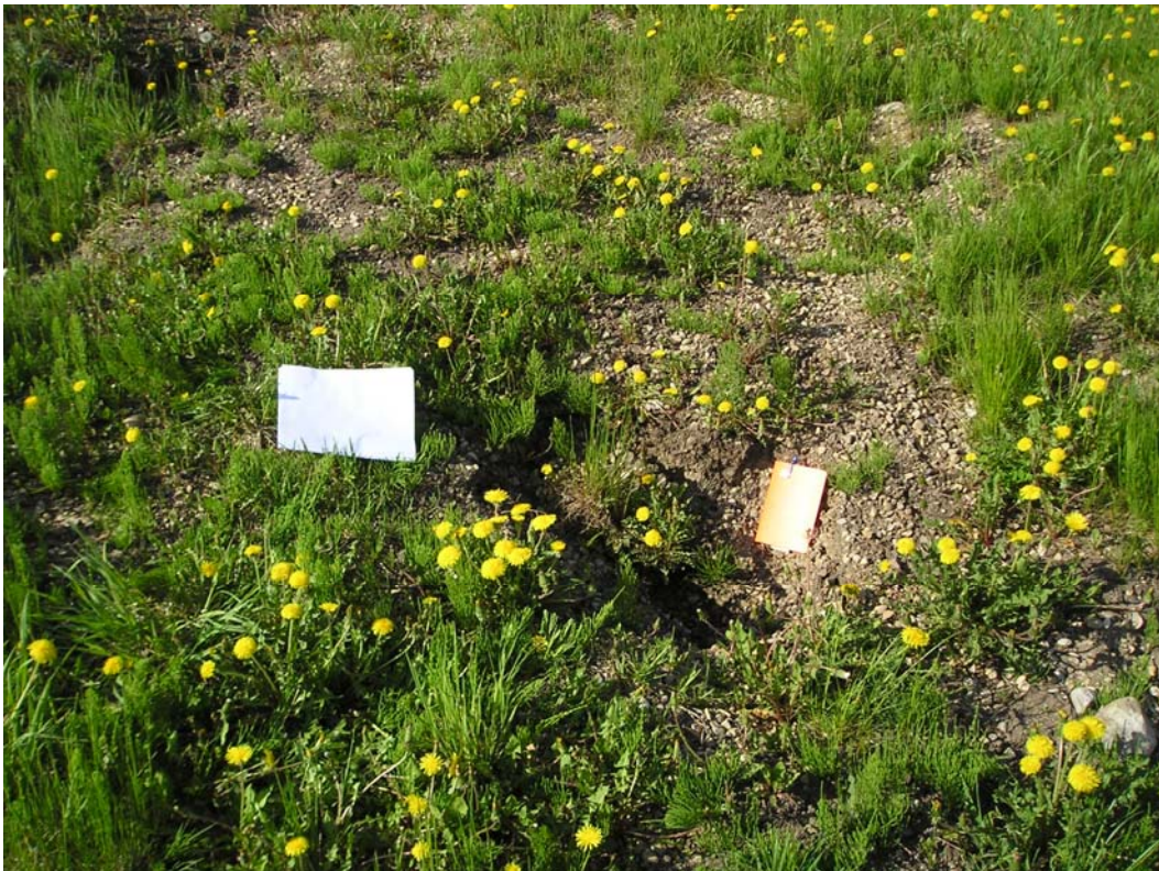
Photo 6 – Sinkholes above culvert outlet at Station 1+680 (looking south). Photos taken May 31, 2005
