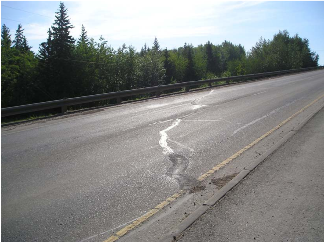
Photo 1 - Looking northeast at west crack.
