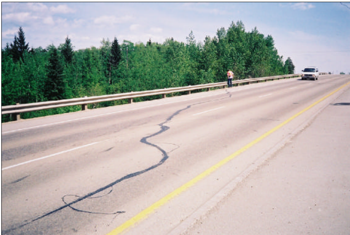
LOOKING NORTHEAST AT EAST CRACKS NEAR STATION 1+860
