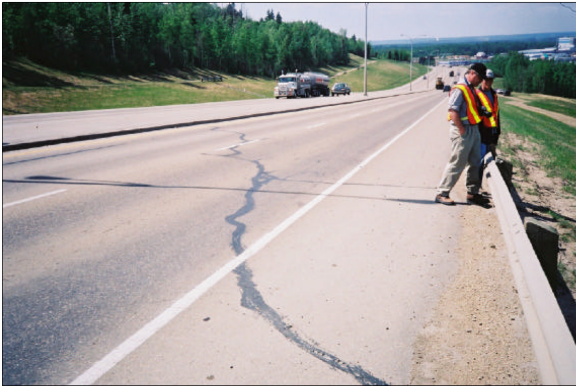
LOOKING WEST AT WEST CRACKS NEAR STATION 1+800
