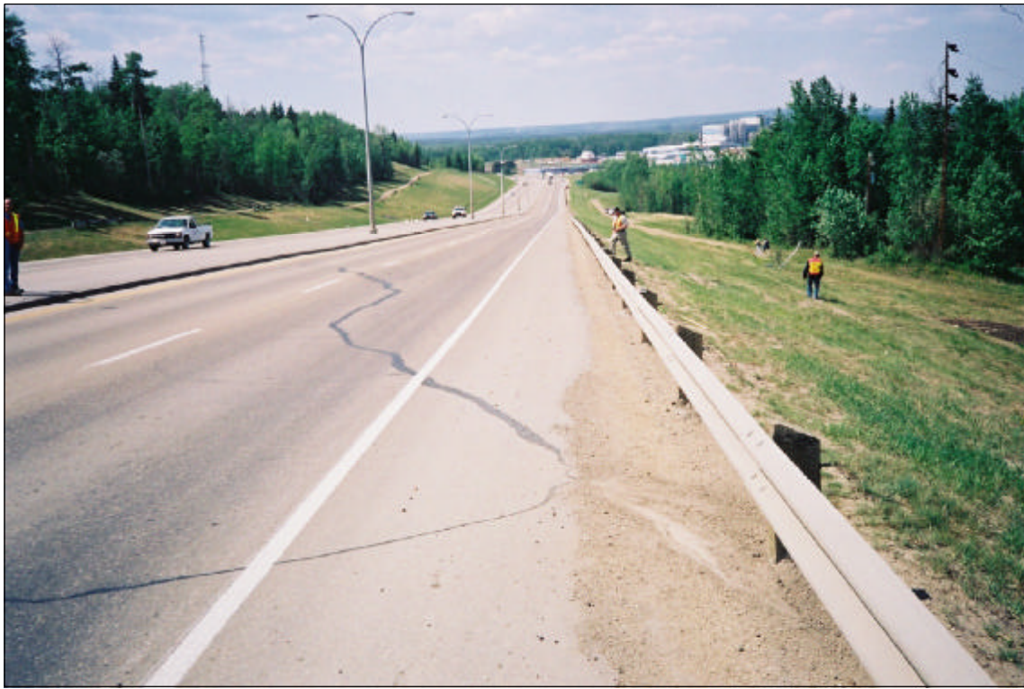
LOOKING WEST AT EAST CRACKS NEAR STATION 1+860
