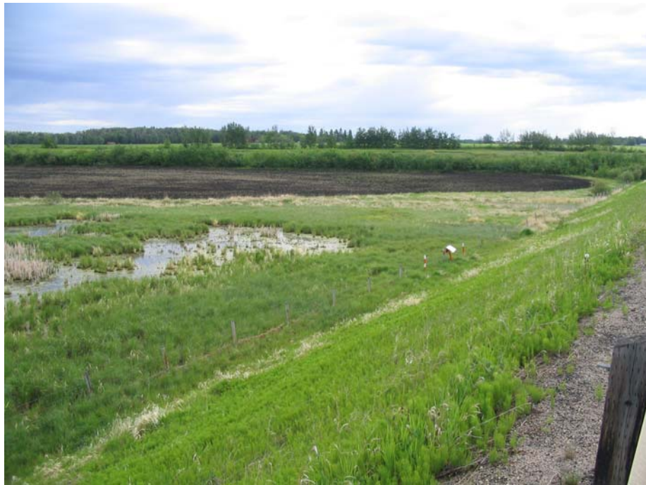
Photo 7 - Looking north - ponded water at toe of north embankment slope, June 7, 2006.
