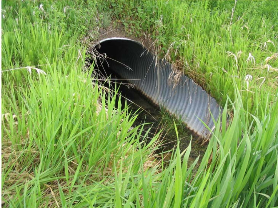
Photo 4 - Looking north at water ponded in culvert, June 7, 2006.
