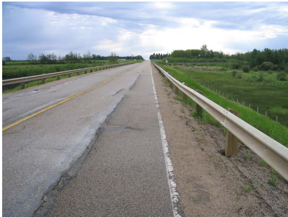
Photo 2 - Looking east possible slide crack, June 7, 2006.
