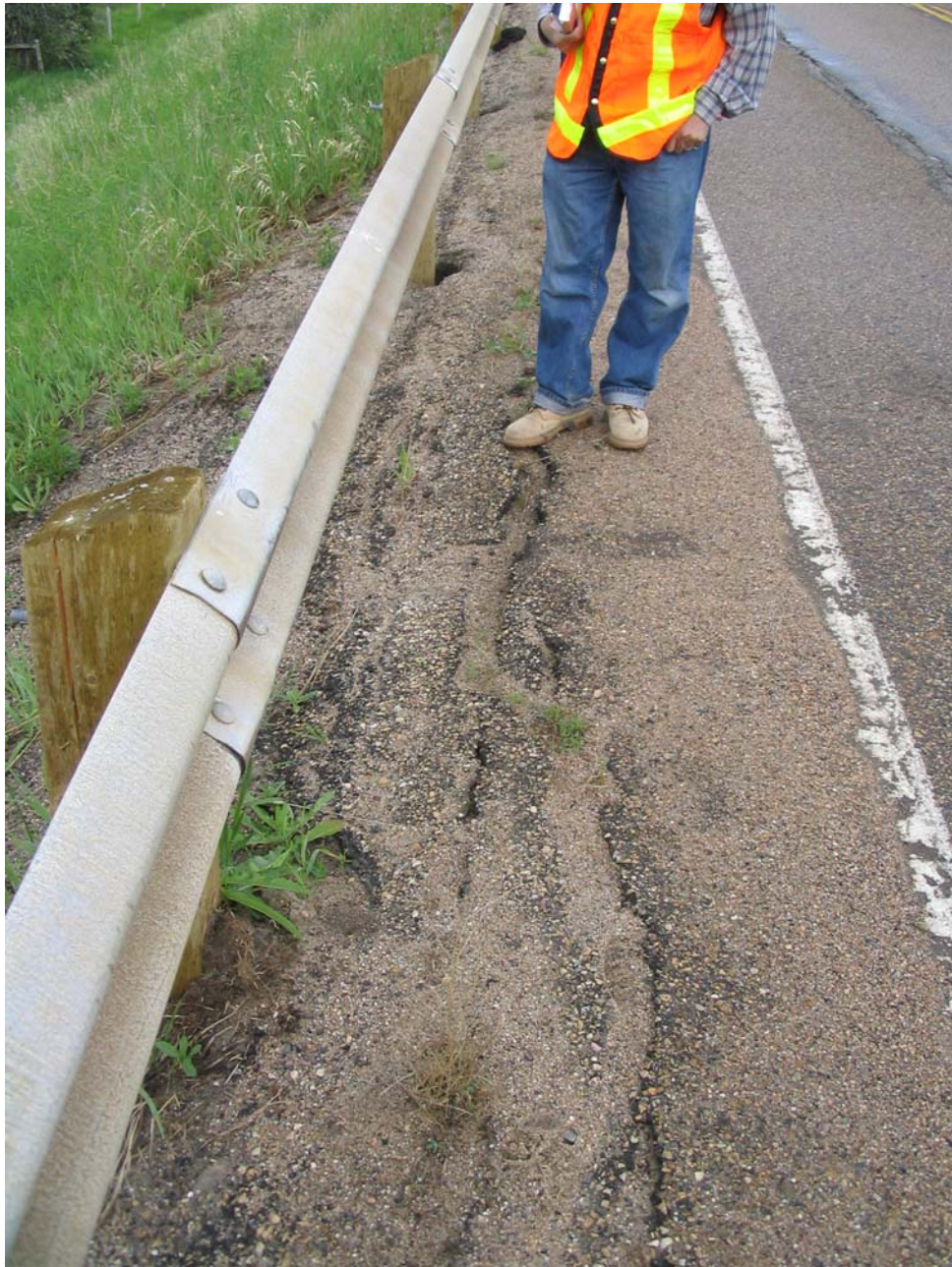
Photo 3 - Looking west at edge cracks over culvert, June 7, 2006.
