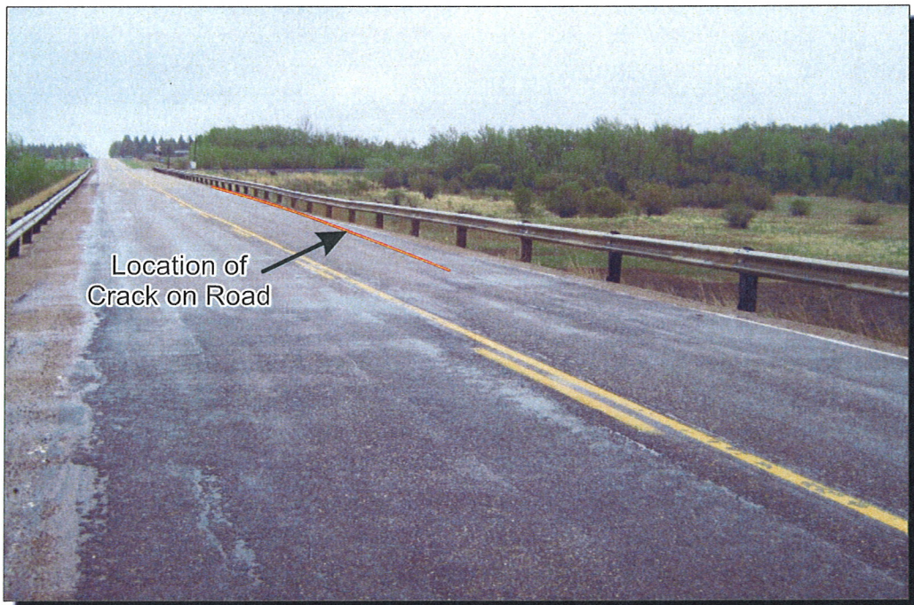
Photo 2 Looking east along Access Road 172; crack present on roadway
