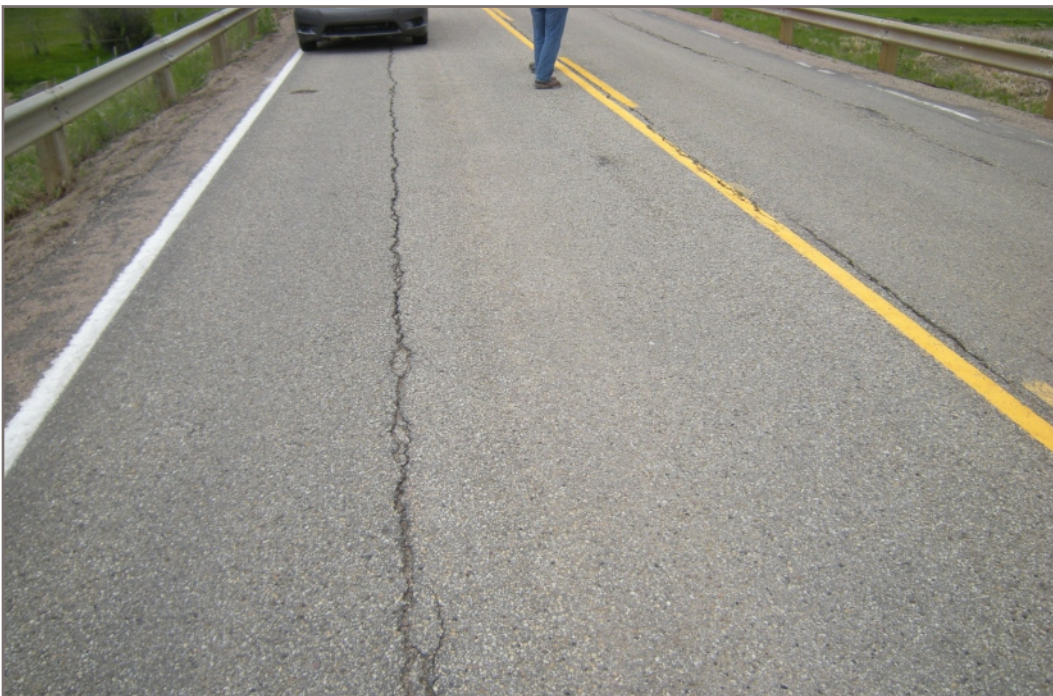
Photo 2: Looking west along Access Road 172; cracks present along roadway
