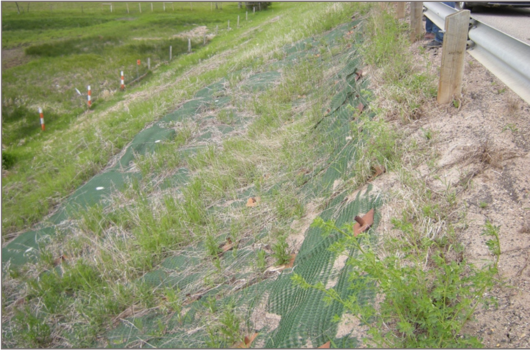
Photo 1: Repaired sideslope requires topsoil and seeding
