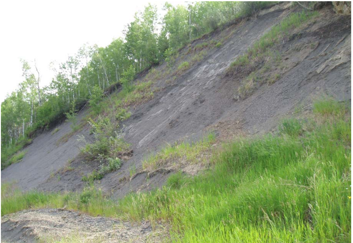
PHOTO 2: Sta. 43+200, Shale backslope and the debris pile
