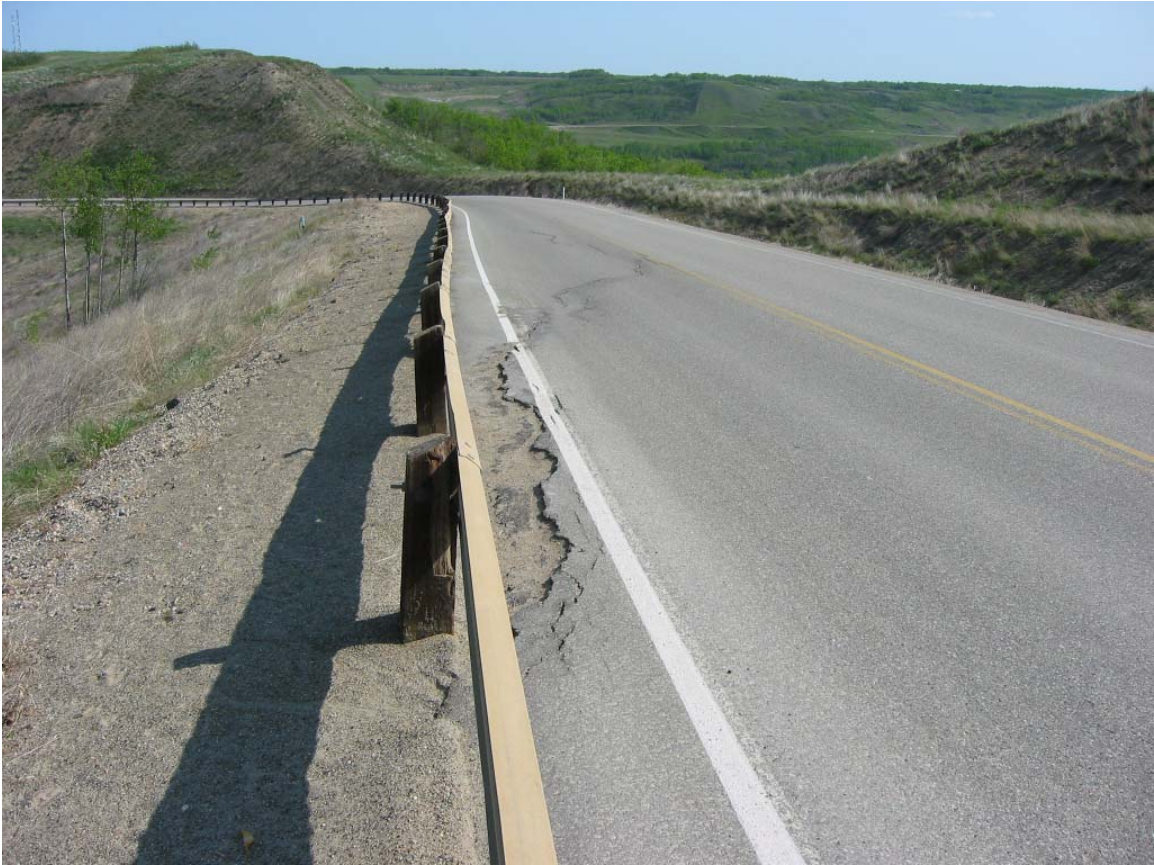
Photo 1: Judah Hill Slide #1, Zone D2, cracks in pavement, May 2003
