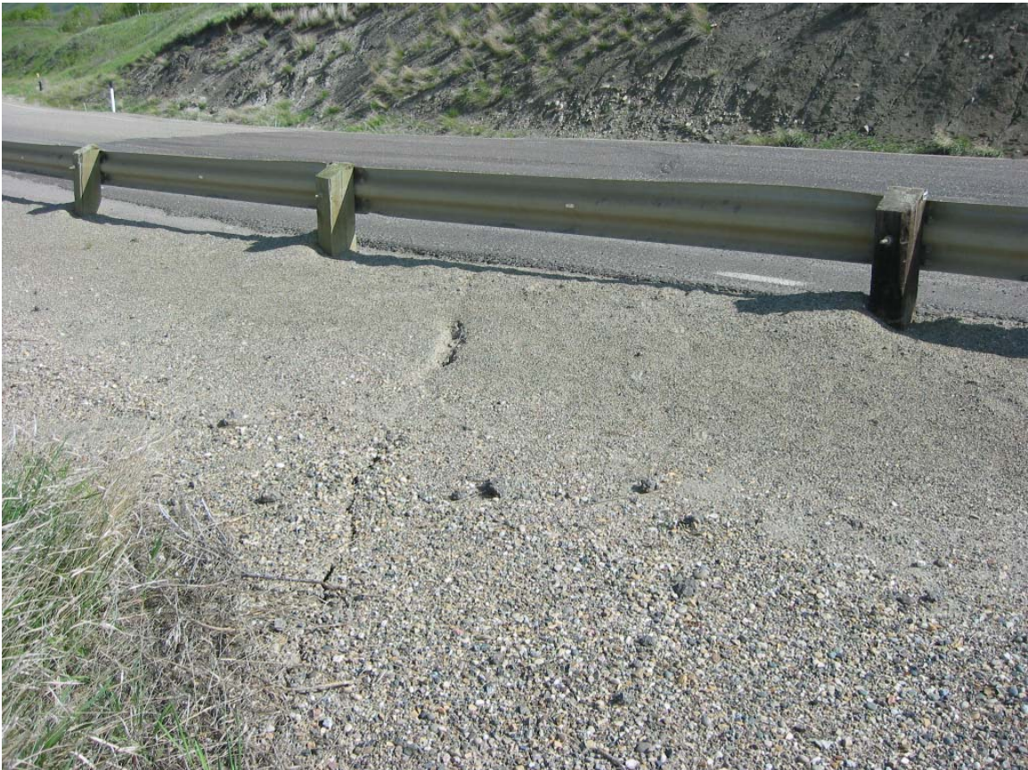
Photo 3: Judah Hill New Slide, cracks in shoulder, pavement patched, May 2003
