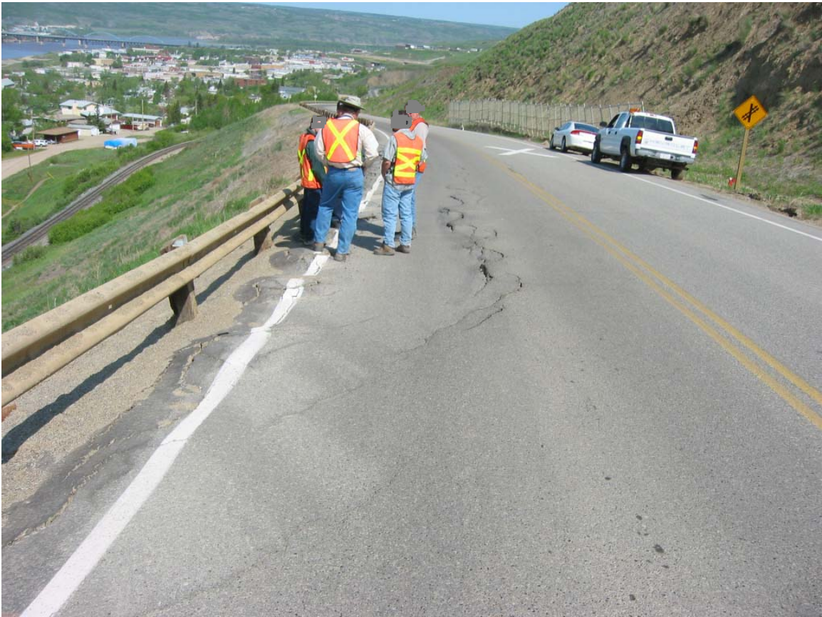
Photo 5: Judah Hill Zone B1, settlement and cracks in pavement, stone columns pushing through, May 2003
