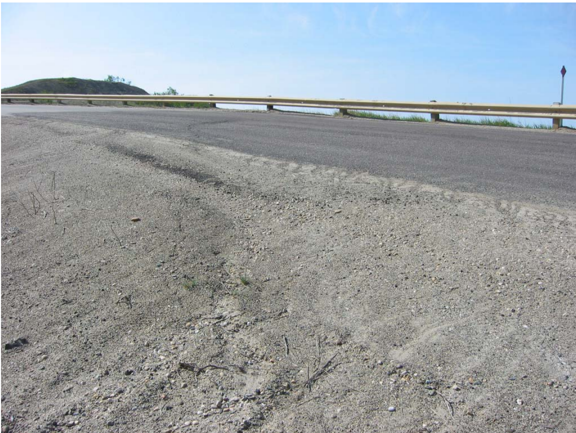
Photo 4: Judah Hill New Slide, scarp, pavement patched, May 2003
