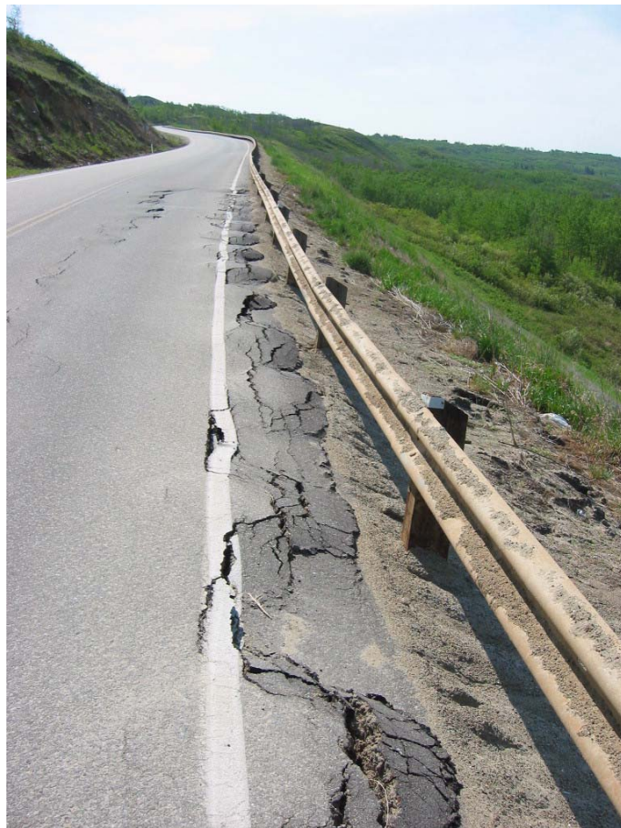
Photo 6: Judah Hill Zone B1, settlement and cracks in pavement, stone columns pushing through, May 2003
