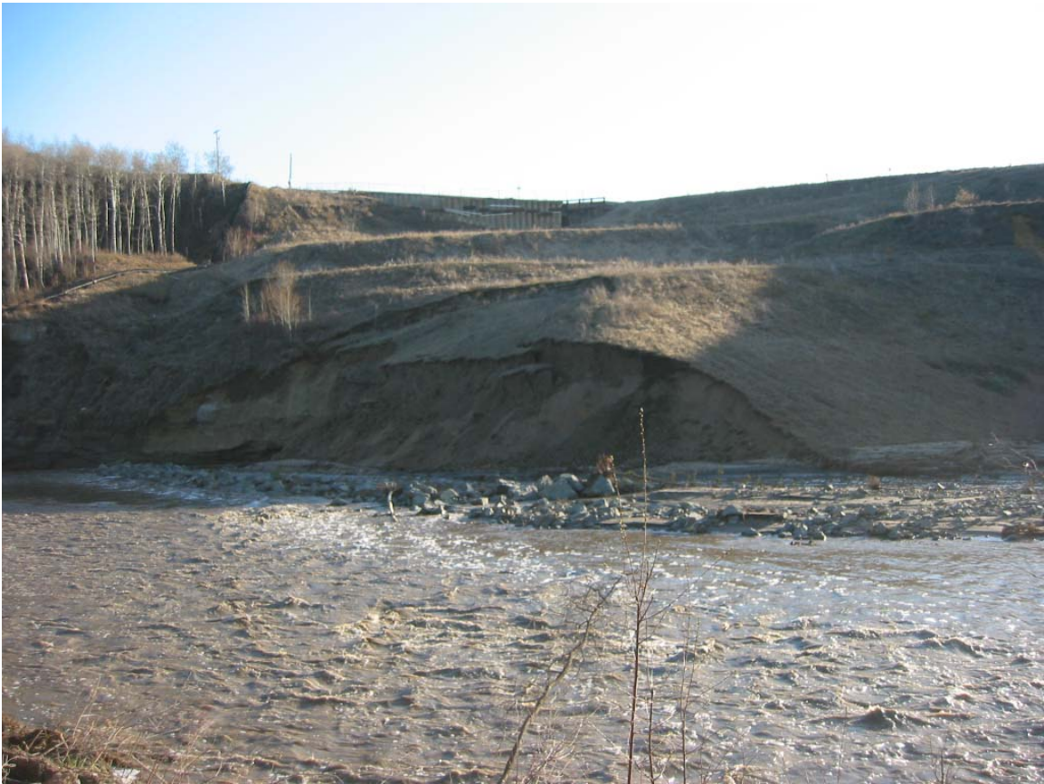
Photo 7: Judah Hill, Slide at Railway Crossing, erosion of buttress, April 2003
