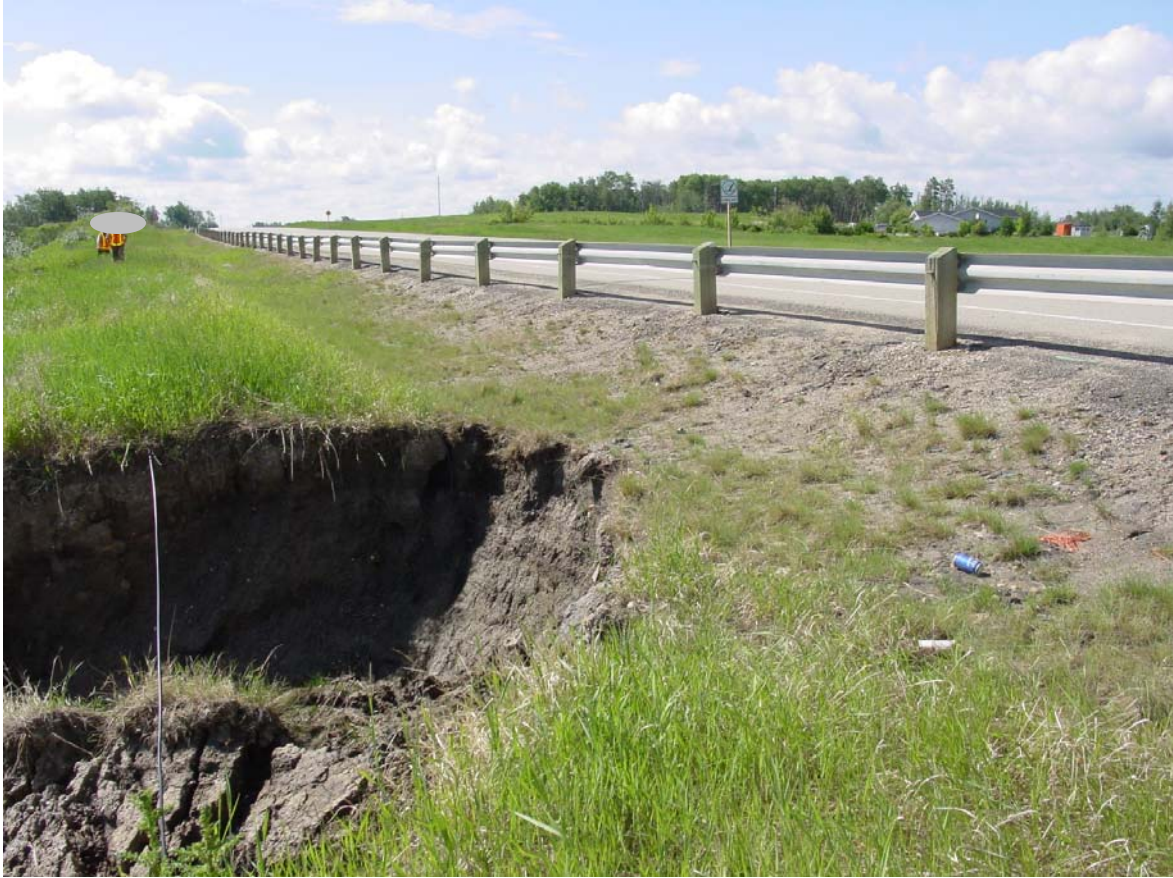
Photo 1 – Slide No 2 – note the barrier has been moved to the edge of the pavement from its previous location just left of the ditch invert. Note the cable dangling across the failure. June 15, 2005
