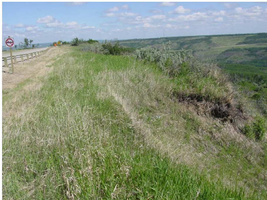
PHOTO 2: Slide 4, showing no significant changes from last year, June 12, 2006.
