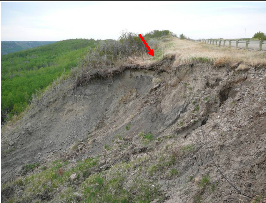
Photo 3. Looking south along the backscarp of Slide 2. There is fresh movement in the backscarp, and erosion due to water draining from the ditch. The vertical offset at the indistinct backscarp south of this slide (arrow) appears to have increased.
