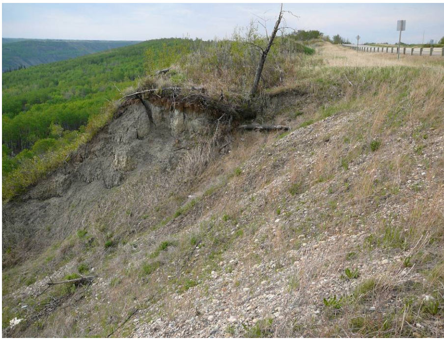
Photo 1. Slide 1 at the north end of the site. No fresh slide movement.
