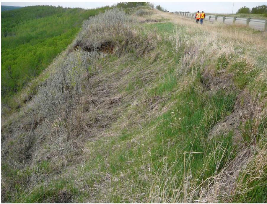
Photo 5. Looking southwards across the backscarp of Slide 3. No fresh movement.
