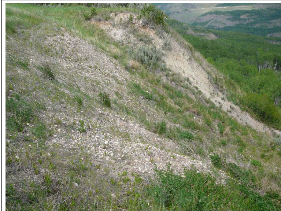
Photo 2. No change in the backscarp of Slide 1 – the repair is working well.
