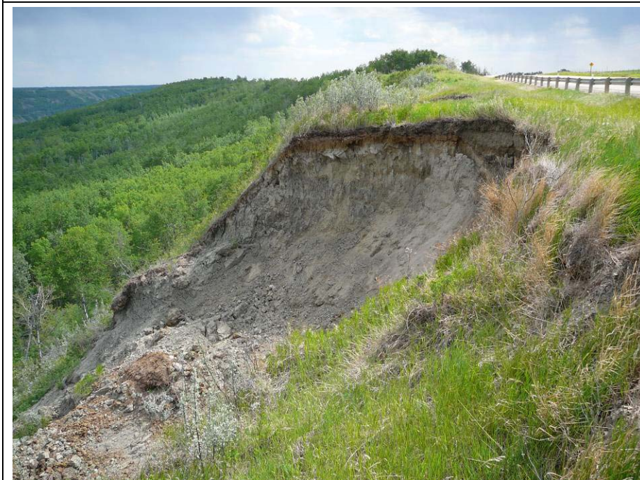
Photo 6. Significant movement on the south flank of the backscarp of Slide 3.
