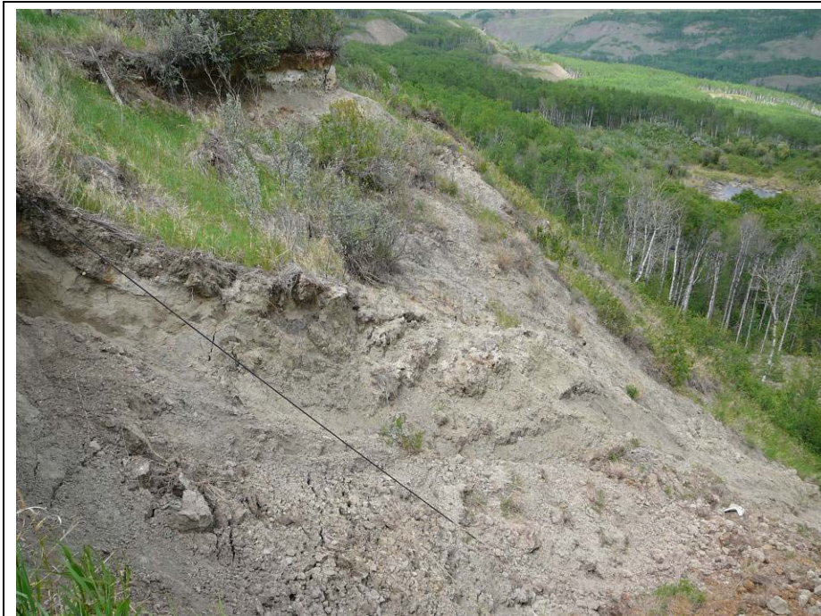
Photo 5. North side of Slide 3. There is not much movement on the north flank of the slide bowl, though significant movement in the remainder of the backscarp, as can be seen in the foreground.
