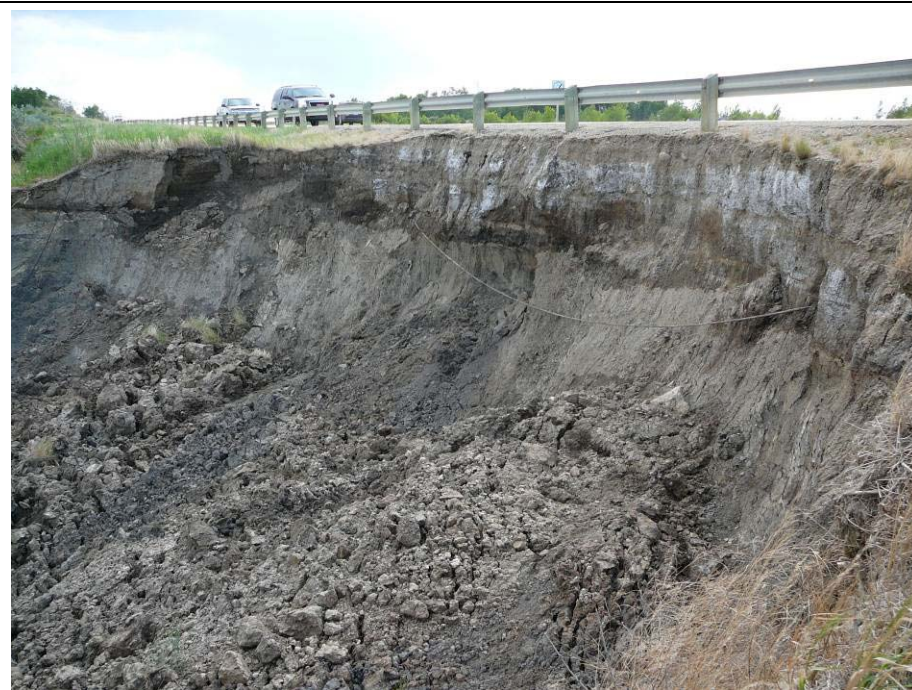
Photo 3. Significant additional movement in the backscarp of Slide 2. The backscarp is now within 0.5 m to 0.75 m of the guardrail – it has retrogressed almost 2 m since 2009.
