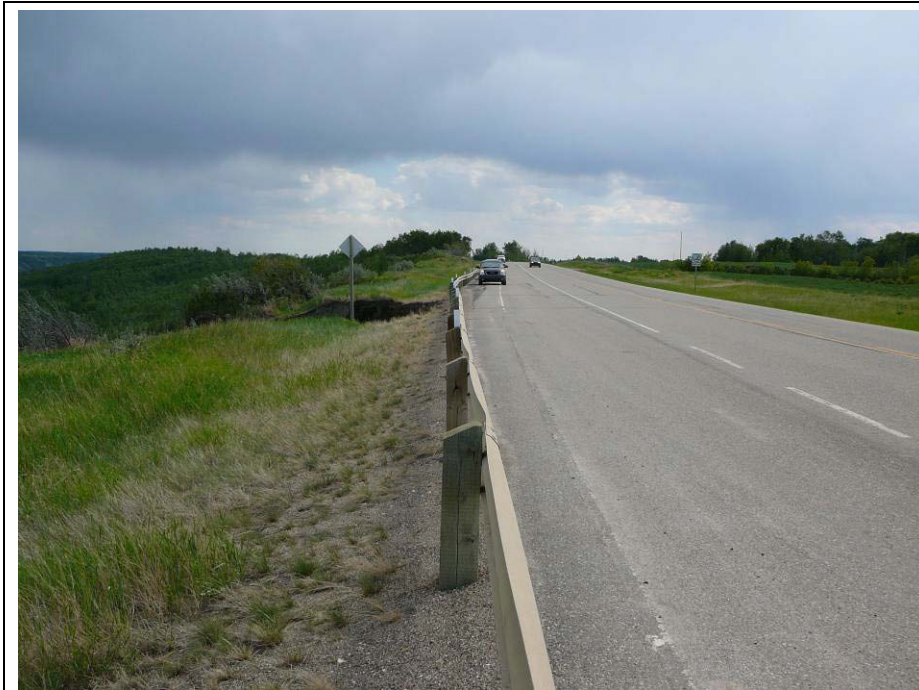
Photo 1. Looking south along Hwy 744 from the south end of Slide 1.
