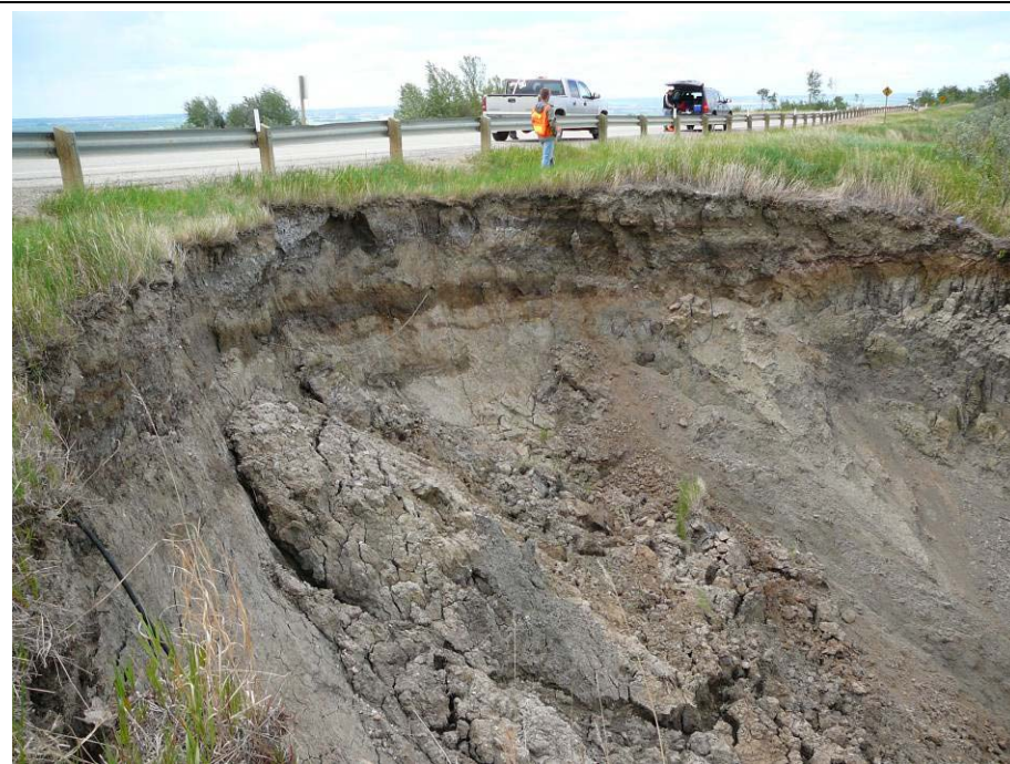
Photo 7. Looking northwards across the backscarp of Slide 4. There has been significant retrogression (1.9 m since 2009) and movement in the slide bowl. The backscarp is roughly 5 m – 8 m high.
