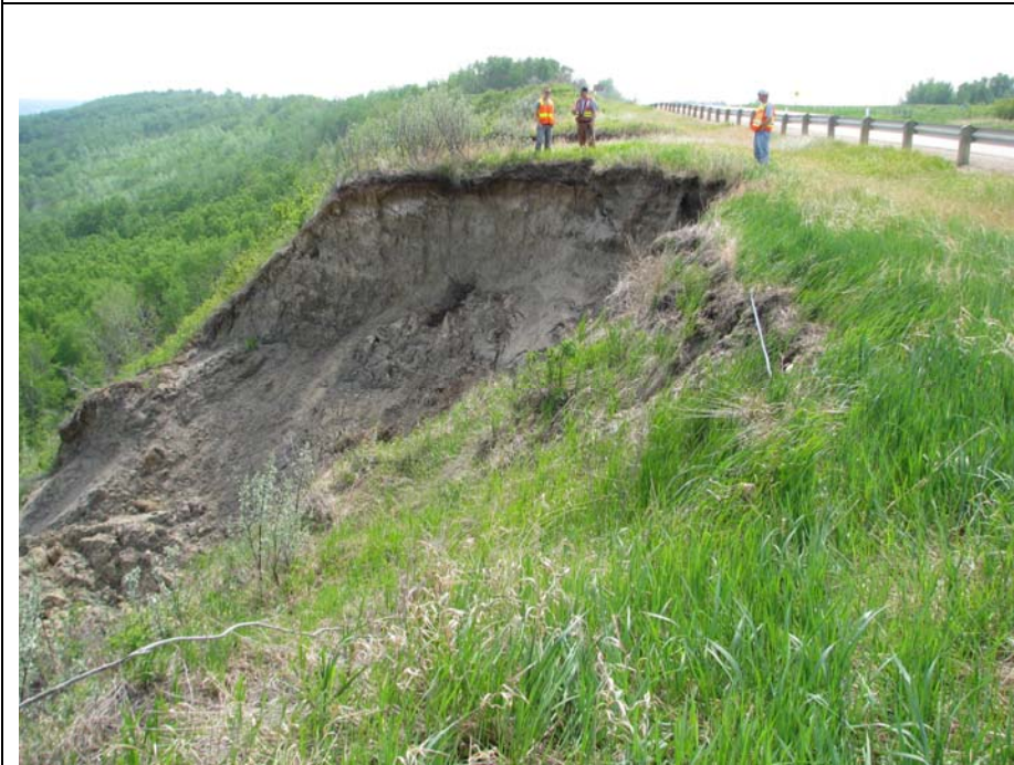
Photo 6. Significant movement on the south flank of the backscarp of Slide 3, now at 4.8 m from guardrail, and about 30 m in width, with fresh cracking and sliding visible,
