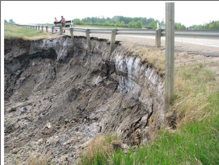
Photo 3. Significant additional movement in the backscarp of Slide 2. The backscarp is now extending as far as 0.7 m past guardrail into pavement, three guardrail posts are now hanging and curve ahead sign is ready to fall over.
