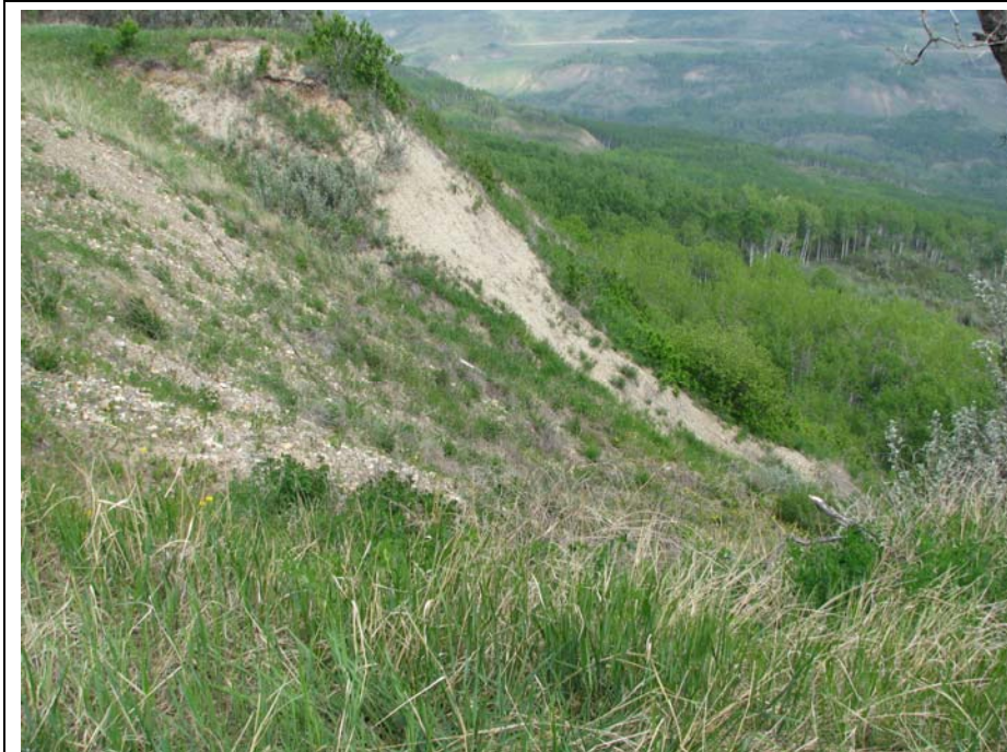
Photo 2. No change in the backscarp of Slide 1 since 2010 – the repair continues to be effective.
