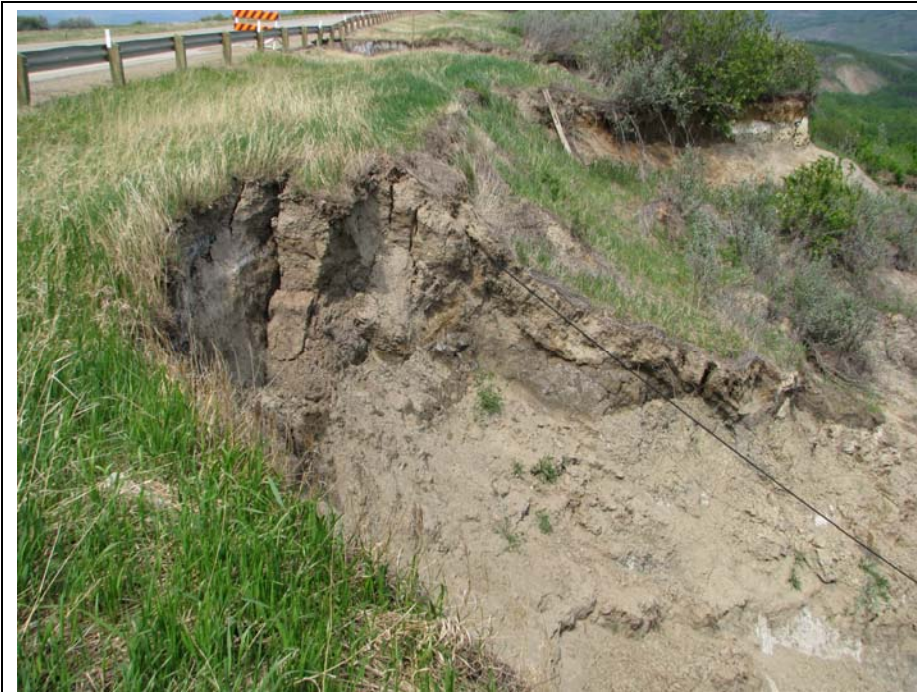
Photo 5. North side of Slide 3. Backscarp geometry is similar to 2010, with slightly more debris flow observed below the backscarp.
