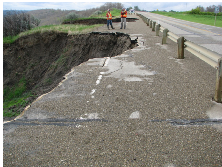
Photo 3. Retrogression movement in the backscarp of Slide 2. The backscarp is now less than 1 m from the new guardrail alignment. Some fresh debris is visible below the scarp and dark seepage stains are also visible from about 1 m to 2 m below the top of the asphalt surface.
