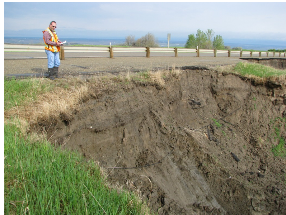
Photo 8. Looking northwards across the backscarp of Slide 4. There has been retrogression since 2012 and some movement in the slide bowl. The backscarp is now at about 3.8 m from the new guardrail alignment (decrease of 0.2 m since 2012).
