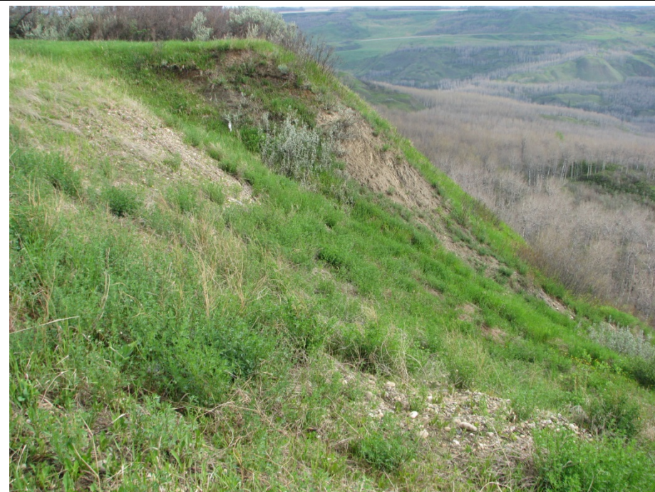
Photo 2. No significant change in the backscarp of Slide 1 since 2012 – the repair continues to be effective.
