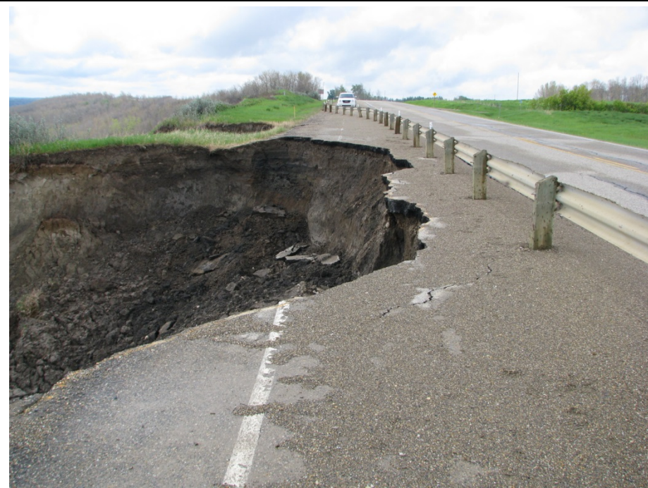
Photo 6. Looking south at Slide 3. Substantial retrogression of the backscarp now at 0.7 m from new guardrail. Dark zones of seepage are visible from 1m to 3 m below the top of asphalt pavement.
