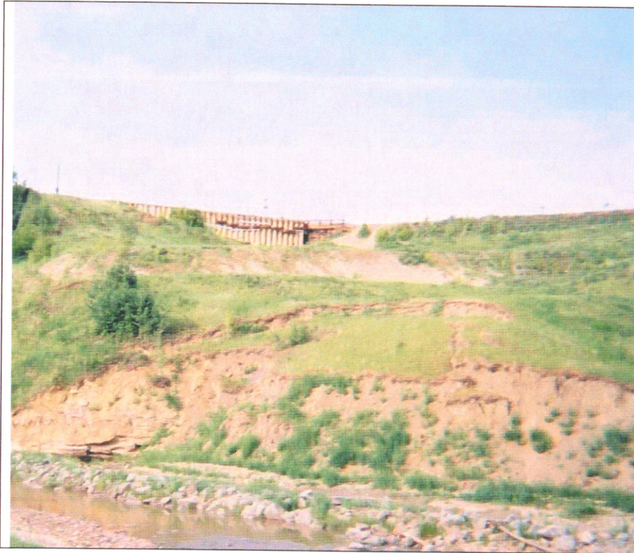
Photo 27. Rail slide taken from the opposite bank of Heart River. Note the bank protection along the toe of the slope and landslide scarps above.
