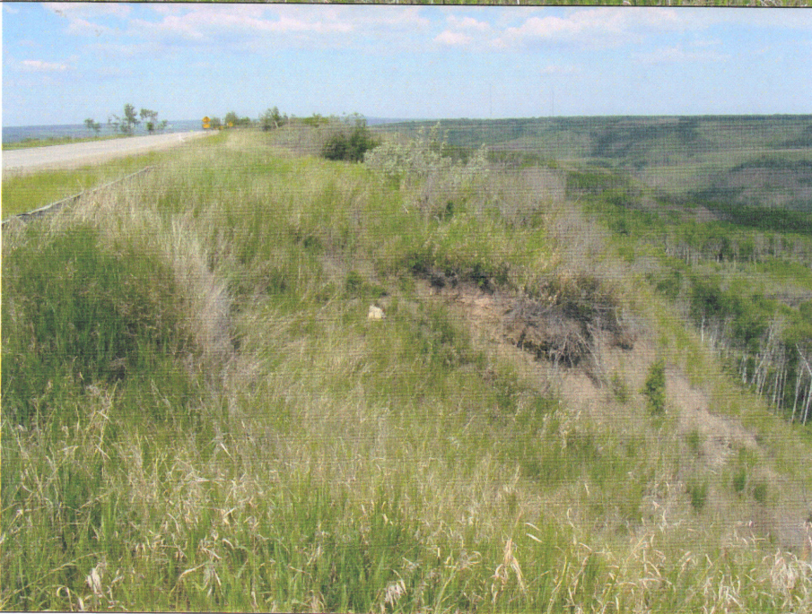
Photo 2. Slide # 3 is the nearest slide to the end of the layby, at the north end of this section. The slide bowl is 35 m wide and the backscarp is within 6 m of the edge of pavement.
