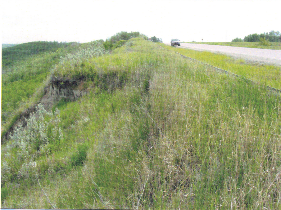
Photo 1. Slide No.4 is the first of several slides along the crest of the slope into the Heart River valley. The slide backscarp is 12 m wide, and roughly 5 m from the edge of pavement.
