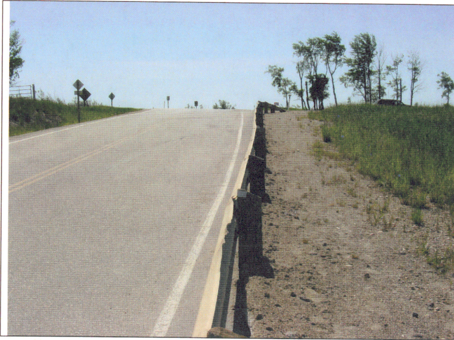
Photo 9. Minor cracking in the pavement at the slide backscarp north of the Lookout.
