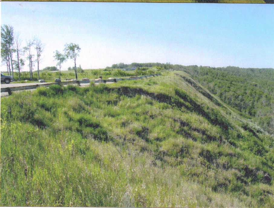
Photo 6. Several slides on the steep slope below the Lookout area. The average slope angle is 38^\circ . The slide area in the foreground is approximately 30 m wide and is currently encroaching on the car park.
