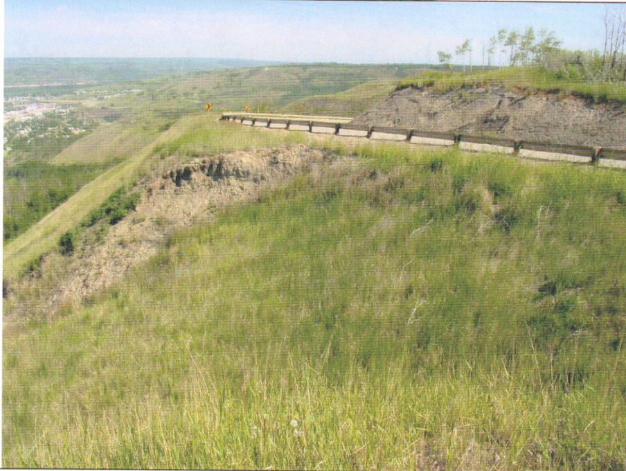
Photo 8. Slide just beyond / to the north of the Lookout. The slide is about 26 m wide, and within 4 m of the guardrail. This is the origin of the slide runout debris in Photo 7.
