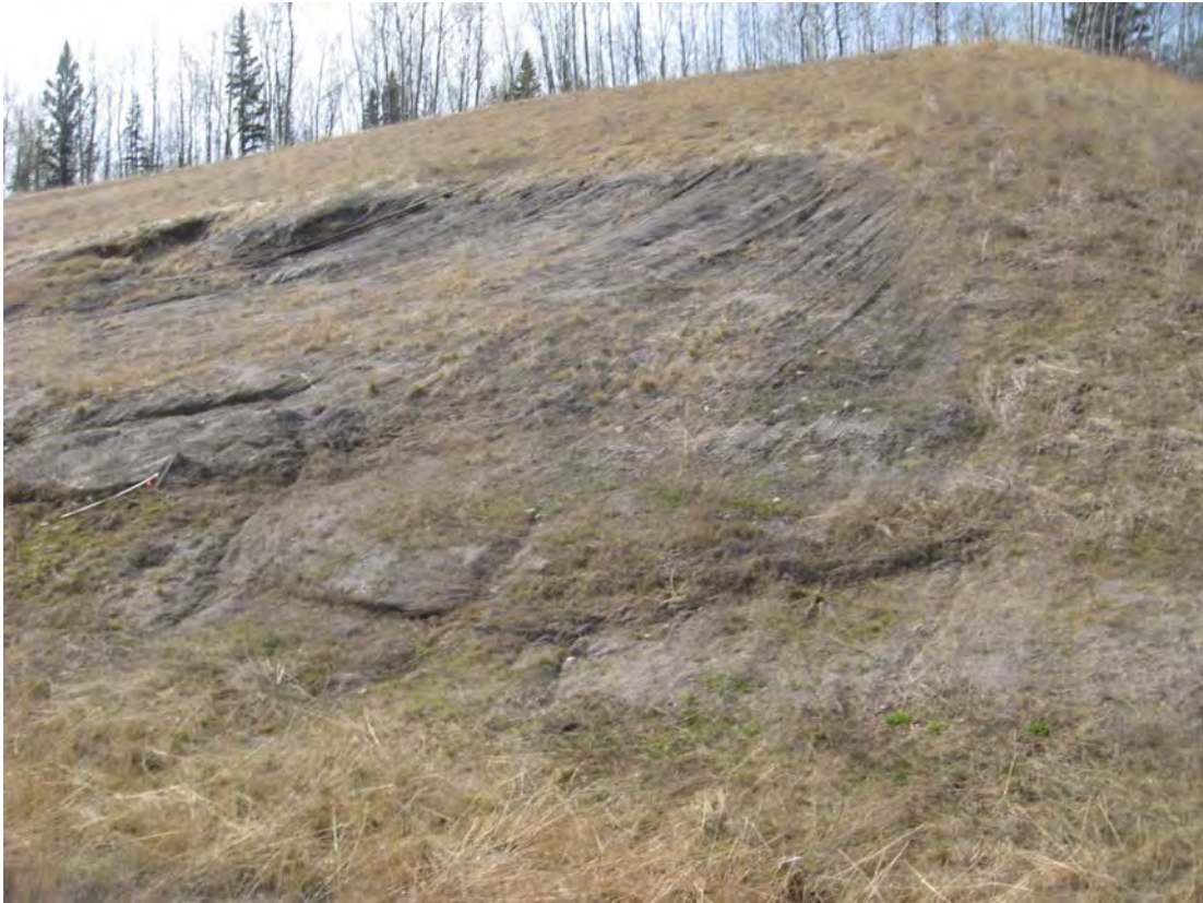
Photo 1 - View of slope failure, looking south.
