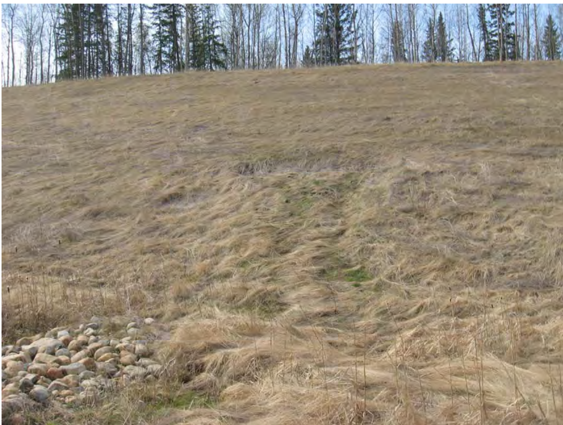
Photo 6 - View of crack located about 60 m east of main slope failure.
