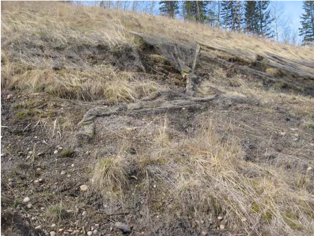
Photo 5 - View of backscarp showing continued seepage, looking southwest.
