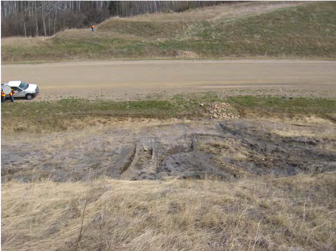
Photo 3 - View of slope failure, looking north.
