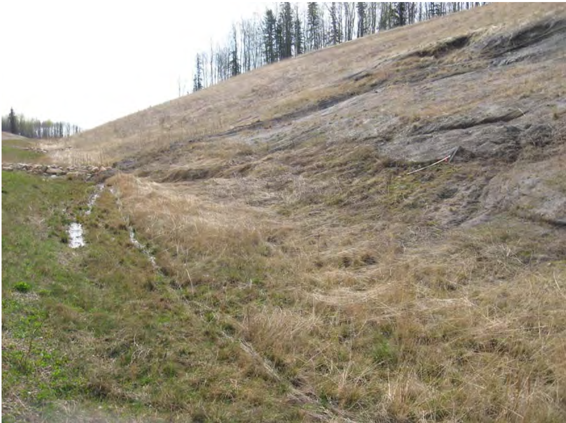
Photo 2 - View of slope failure including toe roll and ditch, looking southeast.
