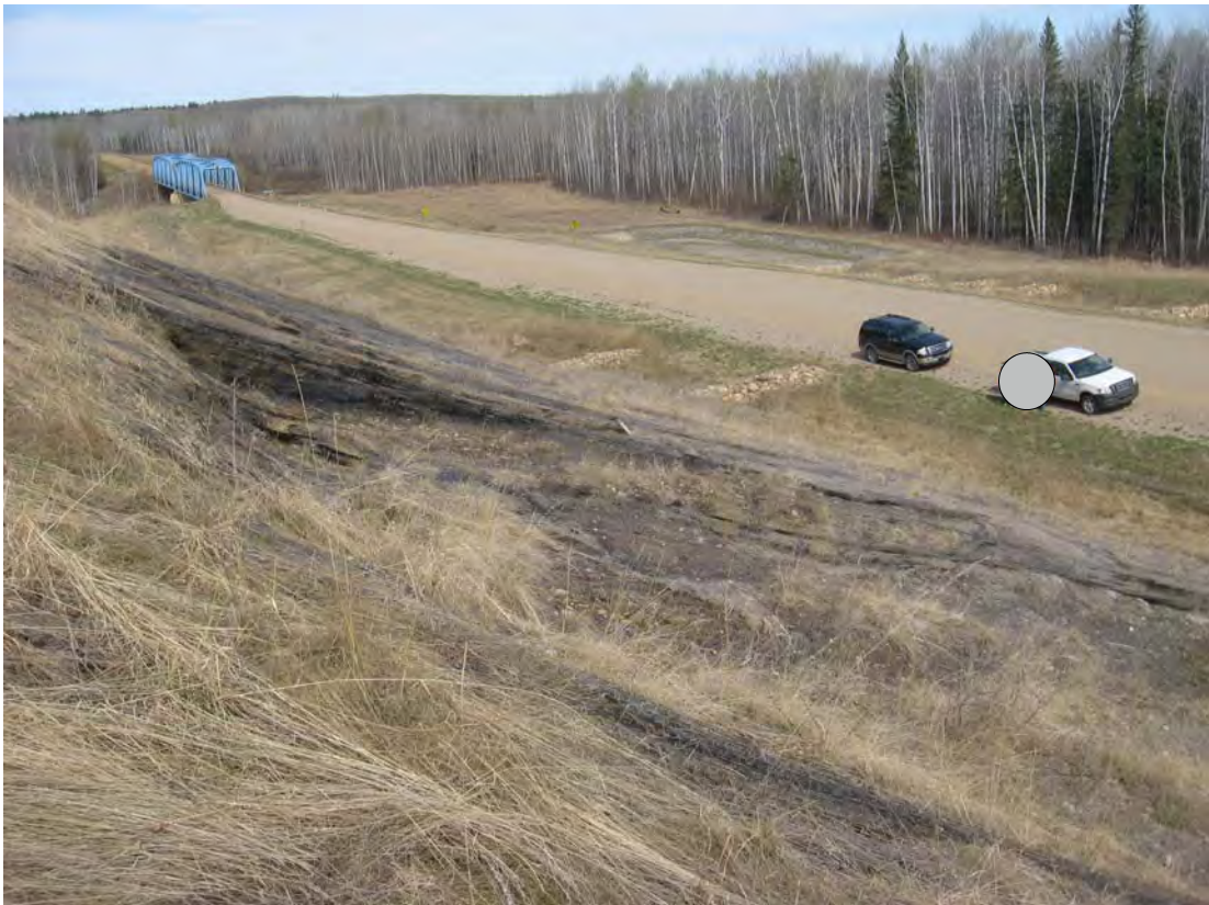
Photo 4 - View of slope failure showing geotextile mesh still in place, looking northwest.
