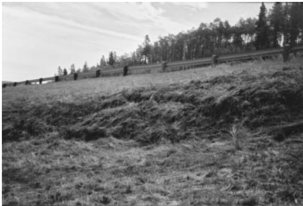
Photo 2 – Oversteepened slope immediately below concrete pile wall along downslope edge of road. Note dip in guardrail.
