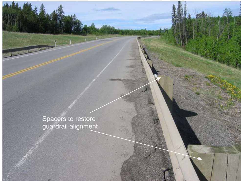
Photo S2-1 (upper left) – May 2006 – Cracking in the westbound lane. The cracking appears to delineate the existing pile wall. This shoulder of the road has been experiencing ongoing cracking and settlement since before the first geotechnical inspection in 2000. The currently-visible cracking has developed through a patch to the road surface that was placed in the summer of 2005.
