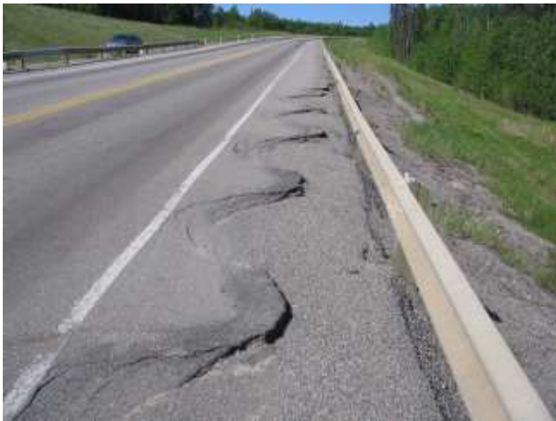
Photo S2-2 – June 2008 (bottom) Closer view of the damage to the road surface. The aperture of the cracks and the amount of down-drop were in the order of 50 mm or even greater at the time of the inspection. Note how the guardrail is relatively low, likely due to ongoing settlement of the ground downslope of the pile wall.
