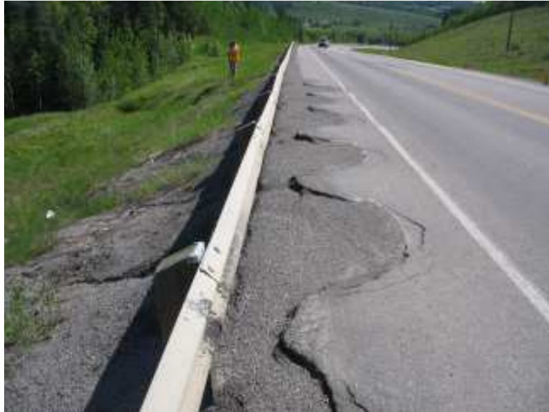
Photo S2-3 – June 2008 (top) Another view of the damage to the road surface, facing eastbound. The apparent east flank of the landslide is visible on the slope face below the road and in the left background of this photo.
