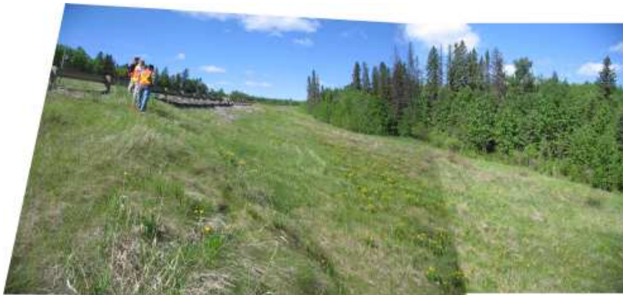
Photo S2-4 – June 2008 (bottom) Facing west along the apparent east flank of the landslide below the highway. The segment of the road surface that shows settlement and cracking and is supported by the pile wall is adjacent to the near-vertical scarp visible on the downslope side of the guardrail in this photo. Each of the SI's on the slope below the highway that are downslope of/within the apparent east and west flanks of the landslide are out of service due to accumulated landslide deformation of the casings. Previous inspections have noted a toe bulge of the landslide area approximately 15 to 20 m into the treed area at the base of the slope.
