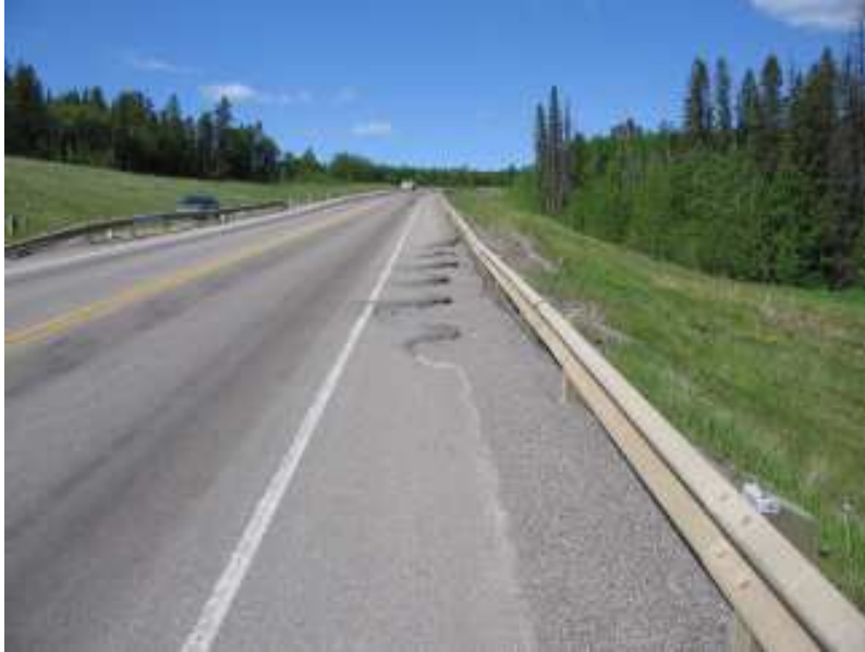
Photo S2-1 – June 2008 (top) Facing westbound across the S2-Priddis site. The settlement and cracking along the north/downslope edge of the highway is visible, along with the corresponding dip in the guardrail. Note how the pattern of damage on the road surface appears to delineate the existing concrete pile wall.
