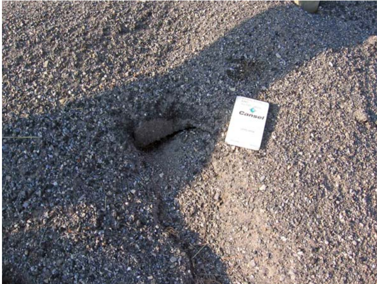
Photo S2-5 – June 2009 An erosion gully that has formed beneath the guardrail and runs towards the downslope. The upslope extent has revealed a pile or other retaining structure.
