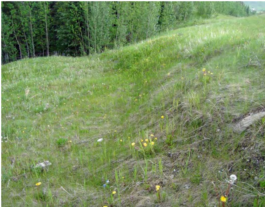
Photo S2-4 (June 2012) – Facing eastbound at the slope below the highway in the landslide area. The slope appears to be in similar condition as was observed in 2011.
