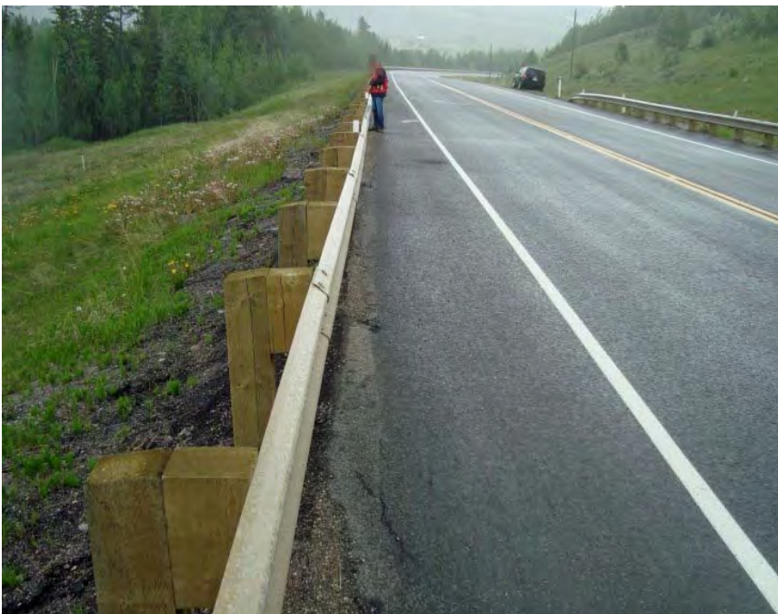
Photo S2-2 (June 2012) – Facing eastbound along the pile wall area. Minor cracking is visible on the shoulder edge of the recent overlay.
