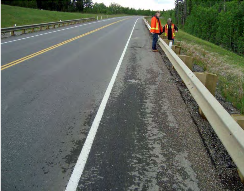
Photo S2-1 (June 2012) – Facing westbound along the downslope edge of the road along the pile wall area. The highway surface here has been recently paved and the guard rail replaced.
