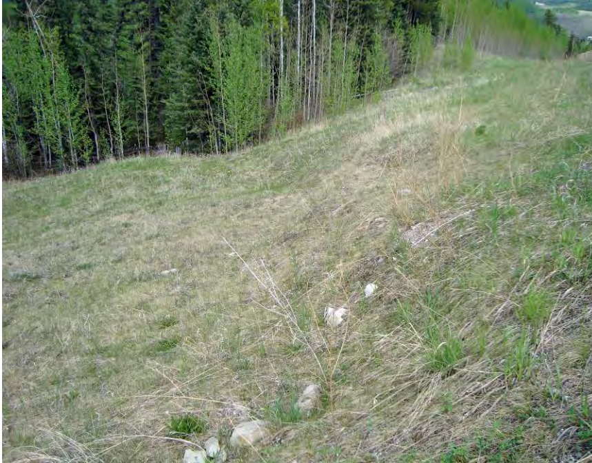
Photo S2-4 (May 2013) – Facing eastbound at the slope below the highway in the landslide area. The slope appears to be in similar condition as was observed in 2012.
