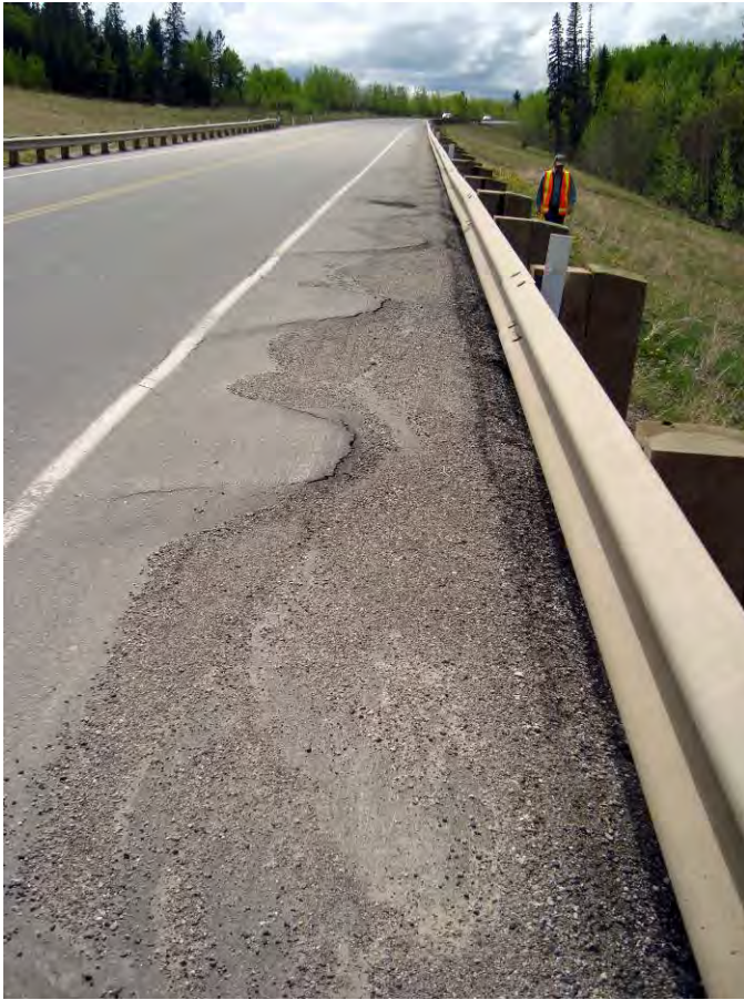
Photo S2-1 (May 2013) – Facing westbound along the downslope edge of the road along the pile wall area. Cracks in the asphalt had formed through the 2013 overlay between the guardrail and white line.
