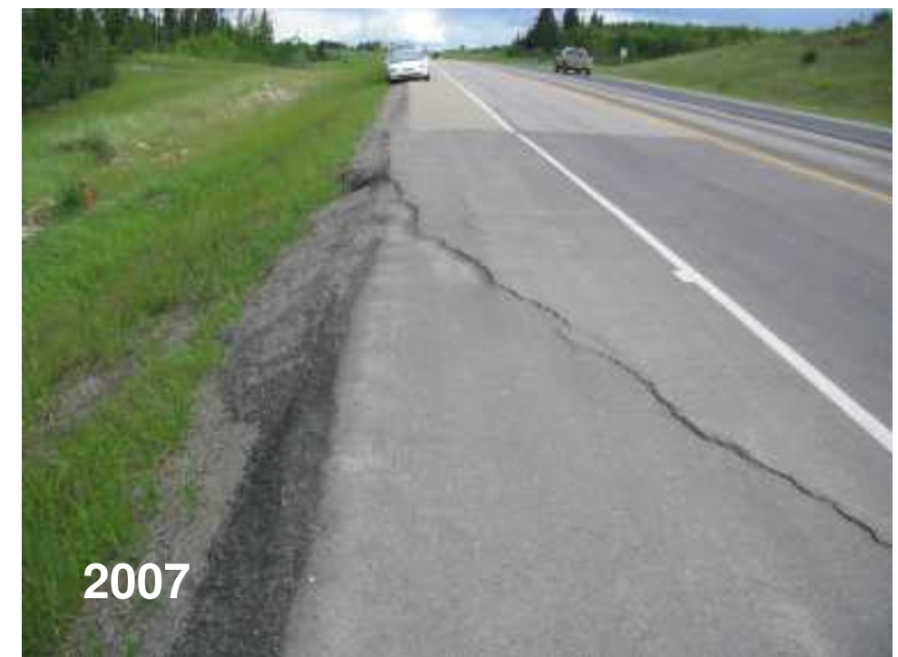
Photo S3-3 – June 2006 (lower left) Cracking and downdrop of the road surface, as seen facing east along the road during the 2006 inspection. The damage to the road shown in this photo was subsequently patched/overlaid and re-formed to the condition shown in Photo S3-2 by June 2007.
