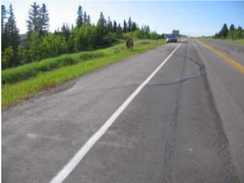
Photo S3-1 – June 2008 (top) Facing southeast across the site, with the apparent circular settlement/landslide headscarp visible encroaching into the northbound lane.
