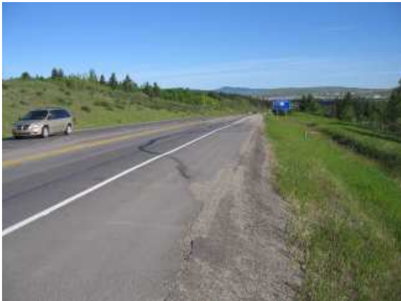
Photo S3-2 – June 2008 (bottom) Another view, facing northwest, of the settlement encroaching into the northbound lane.
