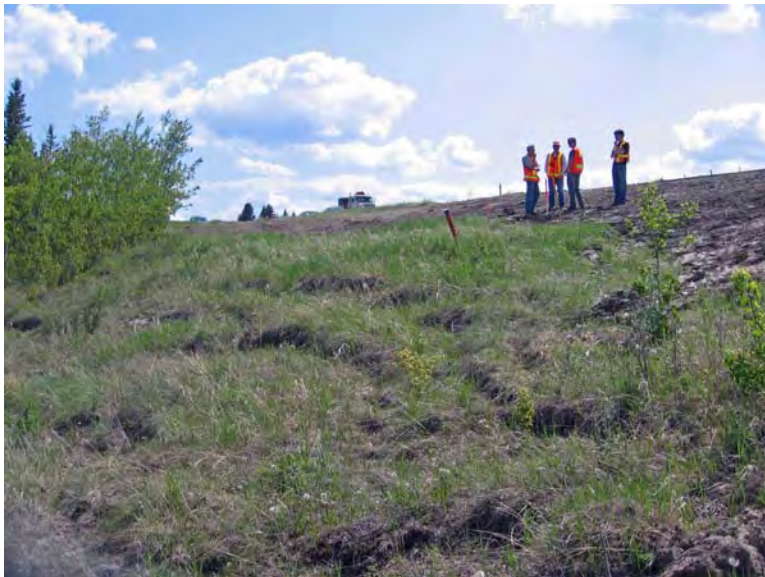
Photo S3-4 – June 2009 Looking towards the south with SI #5 visible. The small scarps appear to be in the same condition as was observed in 2008.
