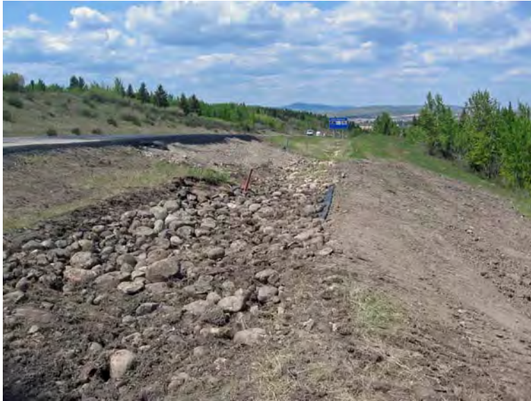
Photo S3-3 – June 2009 A closer view of the repaired ditch area. The 2008 inspection noted a scarp through the ditch berm that has been graded out by the recent repair. Vegetation needs to be established on the freshly graded fill.
