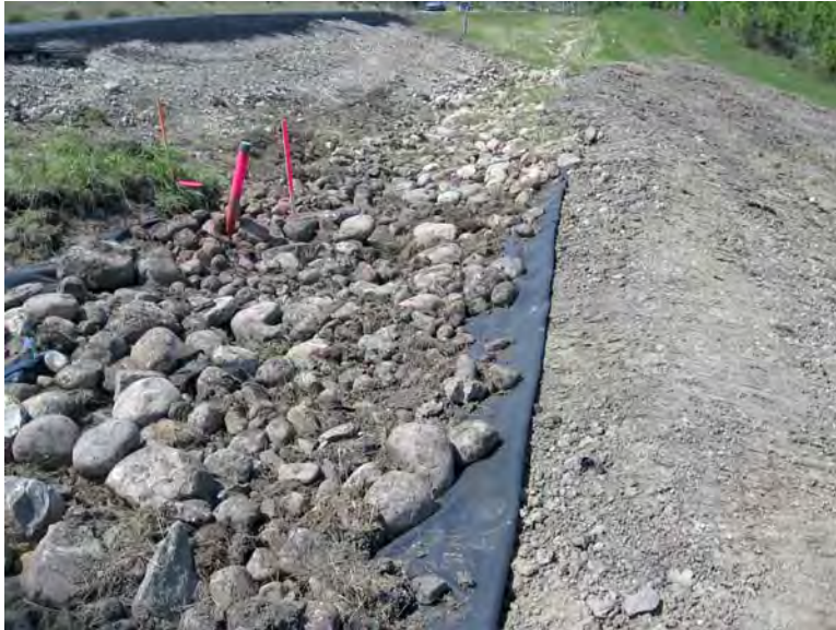
Photo S3-5 – June 2009 A close-up view of the ditch repair with the liner visible. SI #2 is painted on the upslope edge of the ditch.
