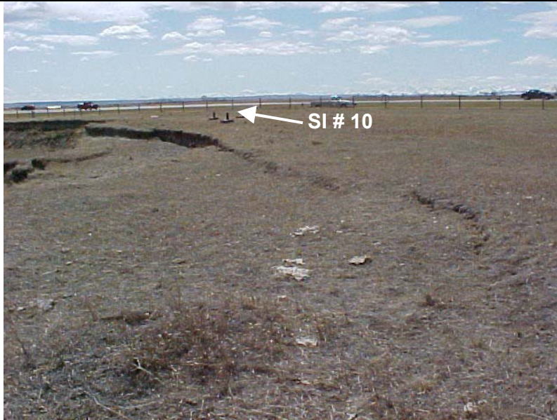
Photo 5 – Facing south towards tension cracks that delineate a new slide block developing on north flank of overall slide. SI #10 in background. (Photo from May 1, 2002).
