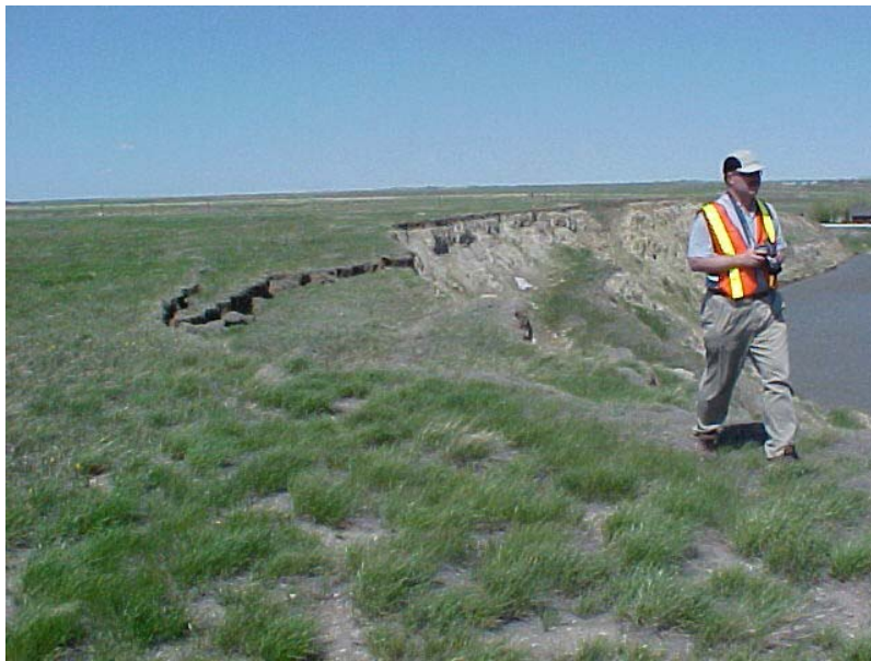
Photo 6 – Facing north from SI #10 towards new slide block developing on north flank of overall slide. (Photo from May 30, 2002).
