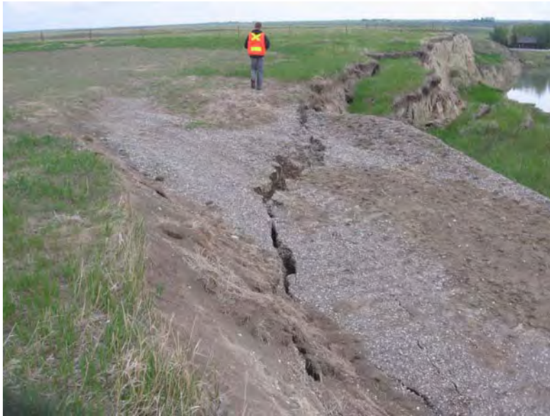
Photo S4-11 (top) – June 2009 Landslide headscarp that has reformed since November 2008 across the uppermost portion of the equipment access trail.
