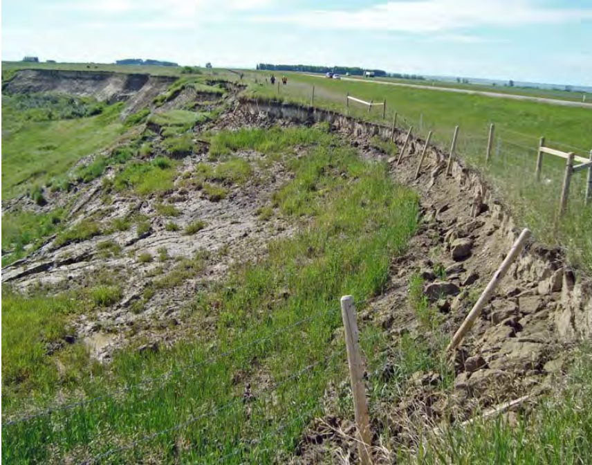
Photo S4-3 (June 2012) – Facing south at the slide area. The instabilities in the upper, steeper portions of the slope are mostly unchanged from 2011 apart from settlement of the larger blocks. Retrogression of the slide continues to occur with large blocks sliding down and adding to the slide mass although at a seemingly slower rate than observed previously.
