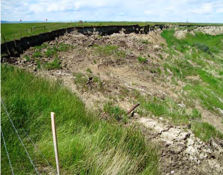
Photo S4-1 (June 2011) – Facing north across the soil nail repair area in 2011, for comparison with 2012 conditions (refer to Photo S4-2).
