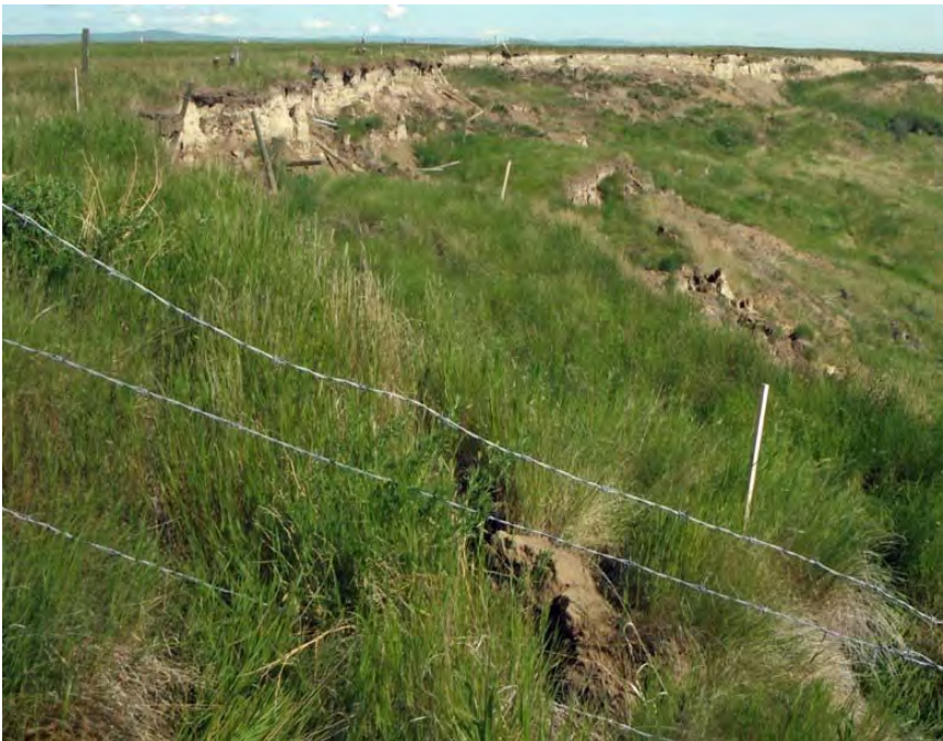
Photo S4-2 (June 2012) – Taken from near the same location as Photo S4-1. Note the displacement of the stake visible in the foreground of the photos, which indicates a retrogression. Continued retrogression at the slope crest, as well as disturbance of the vegetation by soil flows has occurred. Overall the slope appears more vegetated and stable than previous years.
