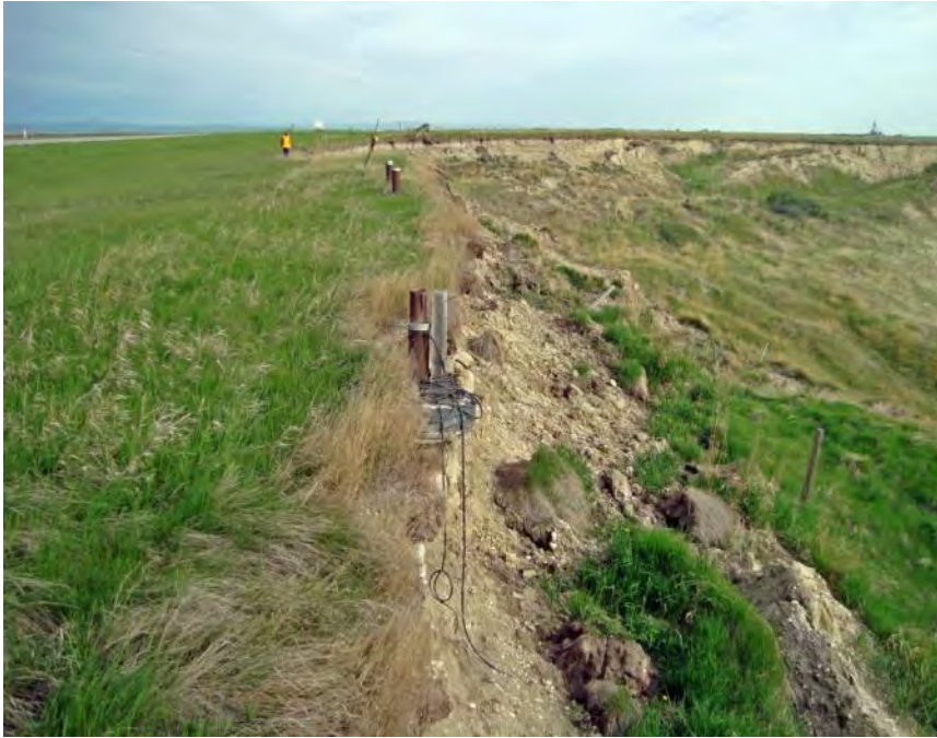
Photo S4-1 (May 2013) – Facing north across the area to the south of the soil nail repair area. The crest is now coincident with the old SI installations from ongoing retrogression.
