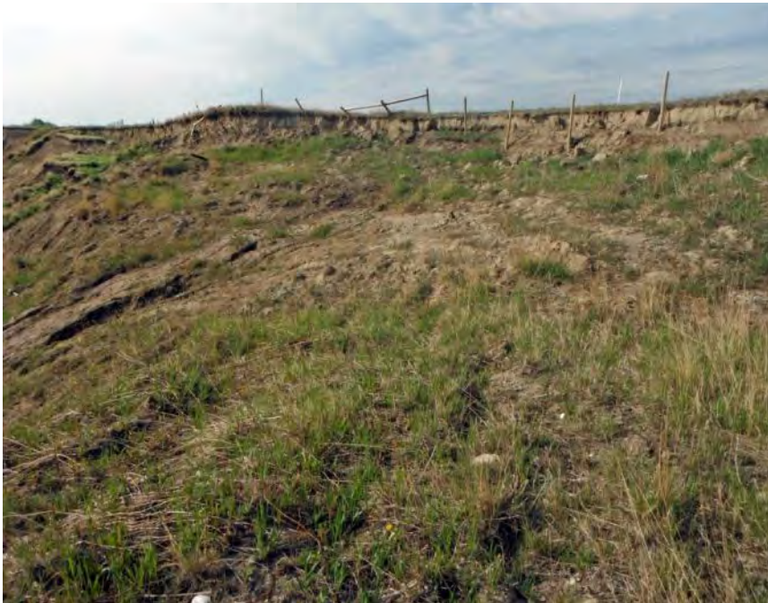
Photo S4-2 (May 2013) – Facing southwest at the slide area within the soil nailed area. The instabilities in the upper, steeper portions of the slope are mostly unchanged from 2012. Retrogression of the slide continues to occur with blocks sliding down and adding to the slide mass although at a seemingly slower rate than observed previously.
