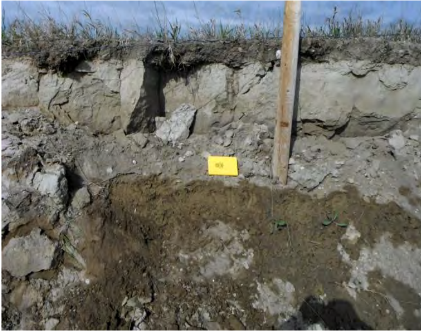
Photo S4-3 (May 2013) – Facing west at the headscarp within the soil nailed slide area. There was visible seepage noted approximately 1 m below the crest.
