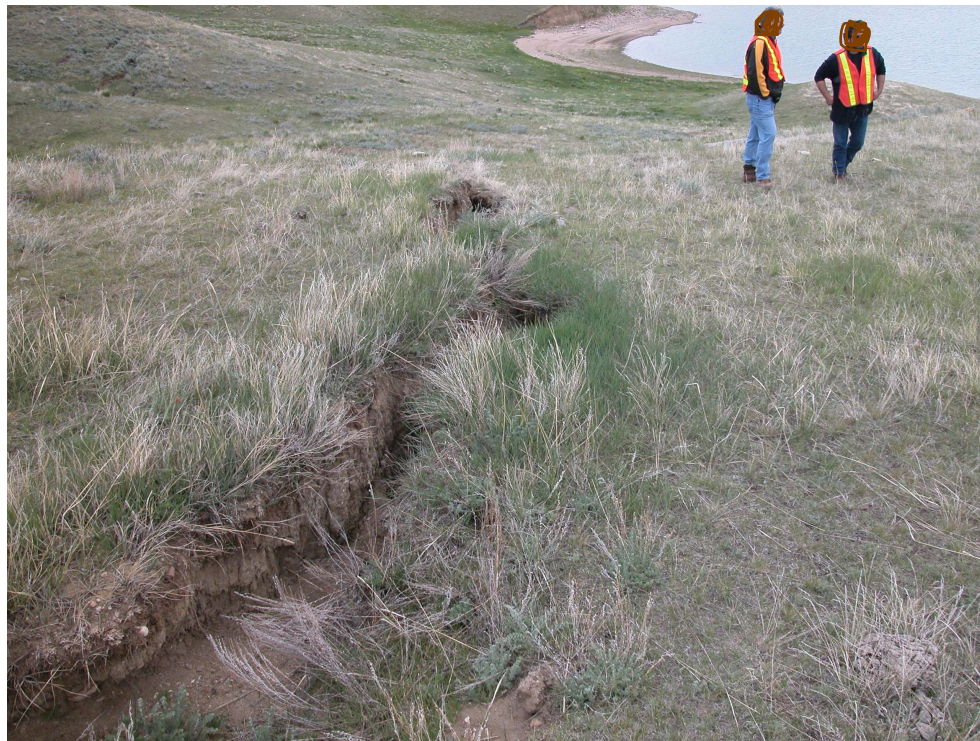
Photo S5-8 (left) – May 2004 – another view of one of the potential new tension cracks on the lower portion of the slope downslope of the highway.
