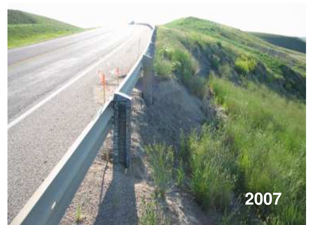
Photo S5-4 – June 2007 (lower right) Another view of the area where the shallow slumping has retrogressed into the paved road surface, with the 2 to 3 m drop in the slope profile adjacent to the highway visible on the right hand side of the photo.
