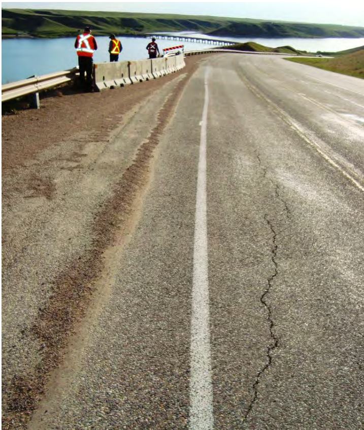
Photo S5-2 (May 2013) – Standing in the eastbound lane facing southwest at the subtle pavement cracking observed northeast of the diversion barriers and retaining wall.
