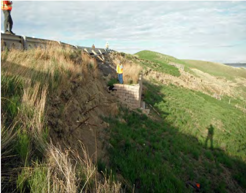
Photo S5-1 (May 2013) – A general view of the site area facing towards the east, illustrating the extent of the wall settlement, undermined guardrail and the exposed soil nails.
