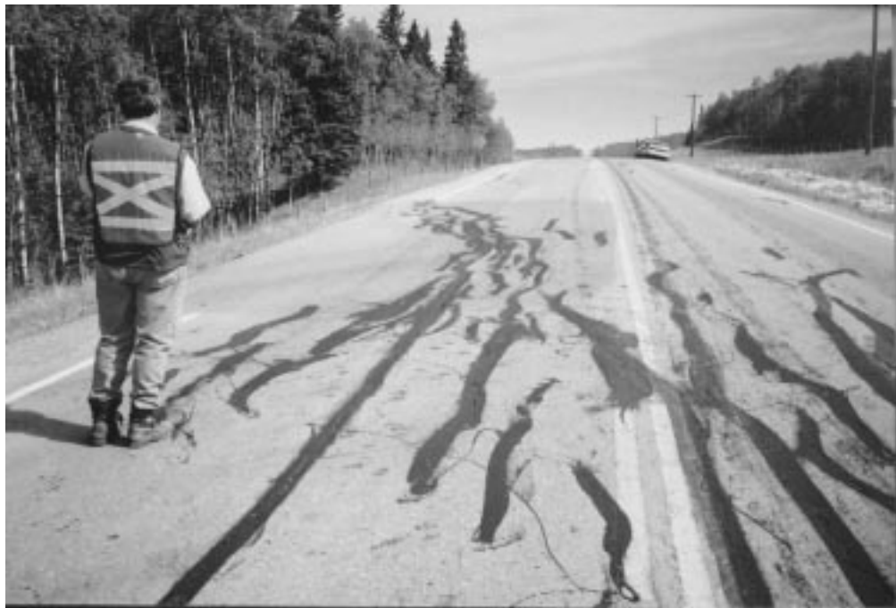
Photo 2 – Facing north across patched and distressed area.
