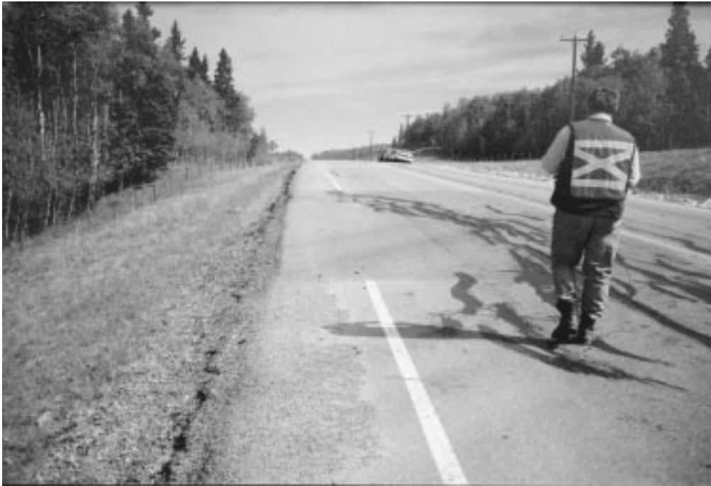
Photo 1 – Facing north across patched and distressed area.
