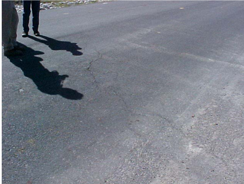
Photo 3 – Fresh cracks in the repaved settlement/cracking area, as seen in May 2002.
