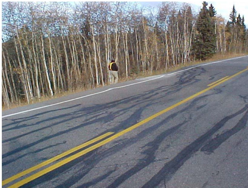
Photo 2 – Another view of the settlement/cracking area before repaving in October 2001.
