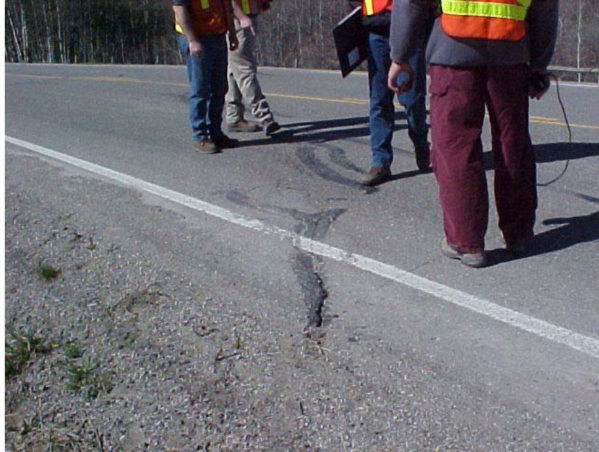
Photo 5 – Another view of the new crack. May 2002 photo.
