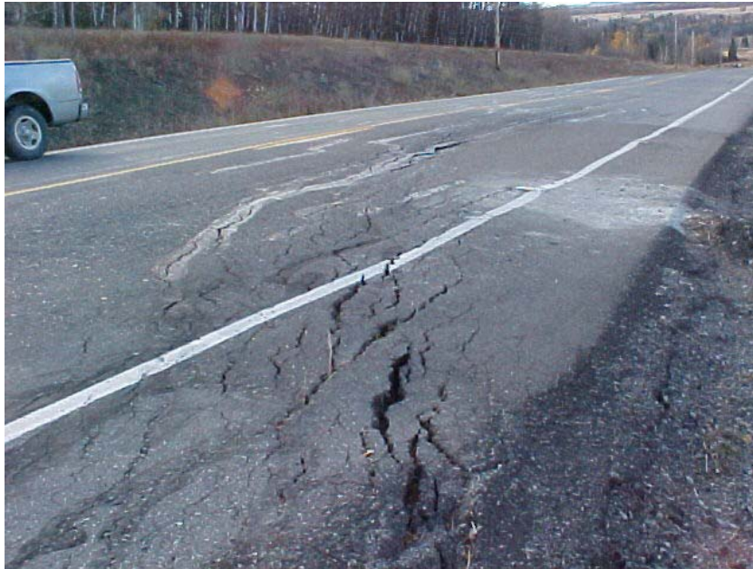
Photo 1 – October 2001 photo of tension cracks in the settlement/cracking area that was previously identified and investigated in the summer of 2001. The rate of movement and cracking in this area appeared to accelerate in the late summer/fall of 2001. This area was repaved in October 2001 after this photo was taken.
