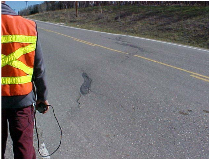
Photo 4 – New crack extending northeast/southwest across the road, approximately 80 m south of the settlement/cracking area shown in Photos 1 to 3. May 2002 photo.
