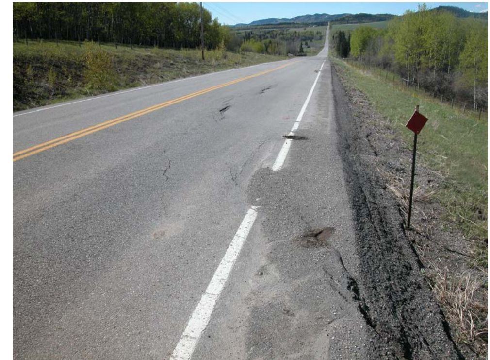
Photo S8-1 (upper left) – May 2004 – cracking and settlement at the north end of the S8 – Fisher Creek site. Similar damage to the road surface has been noted during previous inspections. The SI in BH1 on the west slope below the road is visible (left side of photo). This SI sheared off at approximately 5 m depth between the spring and fall of 2002 and has not been read since. Based on the continued cracking and settlement in this area, slope movement is continuing.
