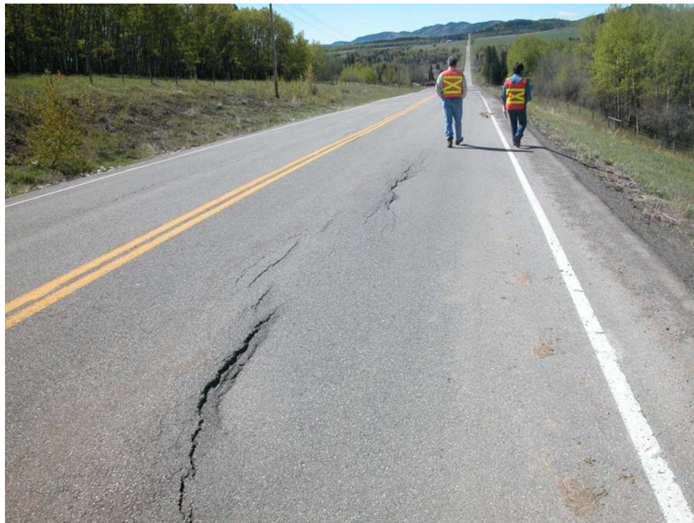
Photo S8-3 (lower left) – May 2004 – a closer view showing the magnitude of the cracking and settlement in the southbound lane at the north end of the Fisher Creek site.
