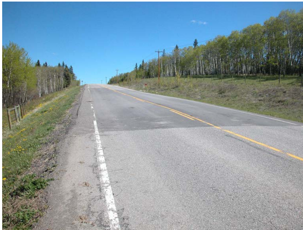
Photo S8-4 (left) – May 2004 – facing north across the south end of the S8 – Fisher Creek site. An arc-shaped crack was first noted in the road surface in this area during the May 2002 inspection and 3 SI's were installed in the fall of 2002 in order to monitor for underlying slope movement that may have caused the cracking. Each of the SI's measured ongoing slope movement towards the west (left side of the photo) at 4 to 6 m depth in the native clay soil underlying the road fill.
