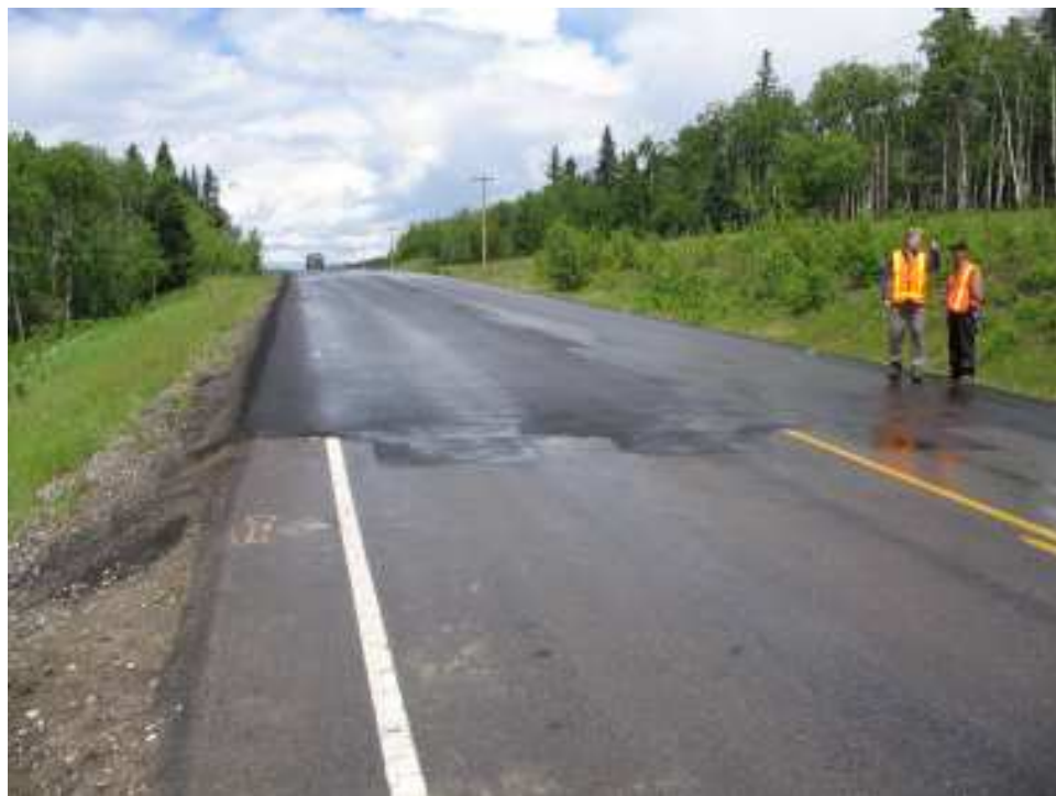
Photo S8-3 – June 2007 (lower left) Facing north across the southern limit of recent overlay around SI 2007-3. The SI at Borehole 2007-3 is marked on the west shoulder of the road, on the left side of the photo.
