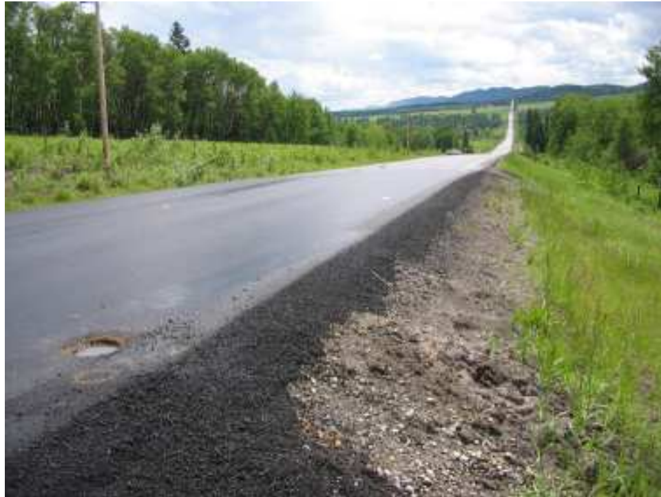
Photo S8-5 – June 2007 (upper left) Facing south across the recent overlay with the SI at Borehole 2007-2 visible in the left foreground of the photo. The thickness of the recent overlay in this area was approximately 50 mm.
