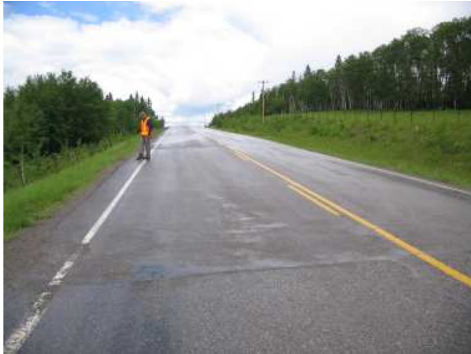
Photo S8-1 – June 2007 (upper left) Facing north from the central portion of the site with the recent overlays on the road surface visible.
