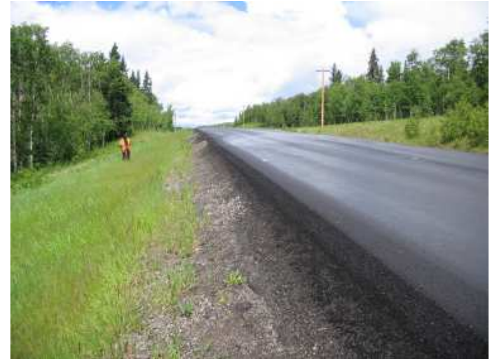
Photo S8-6 – June 2007 (upper right) Another view of the recent overlay area around the north end of the site. Based on the cross-section exposed at the edge of the road, the thickness of the overlay seemed to range between 25 and 50 mm. Note the steep drop-off on the west side of the road (left hand side of the photo).
