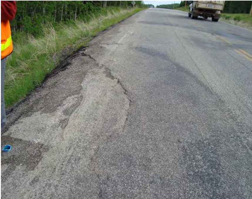
Photo S8-1 (June 2012) - Facing north along the west edge of the road surface at the north end of the site. This area had the most significant cracking following a similar pattern as has been observed during previous inspections. The road surface has been smoothed over from recent milling work.
