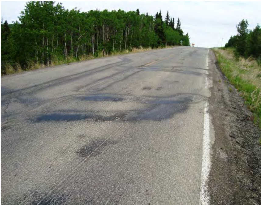
Photo S8-2 (June 2012) - Facing north from the middle of the site. The amount of additional cracking in the road surface is relatively minor, and follows a similar pattern as has been observed during past inspections.
