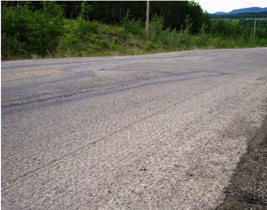
Photo S8-3 (June 2012) - Facing southeast at the visible settlement in the upslope lane at the north end of the site.
