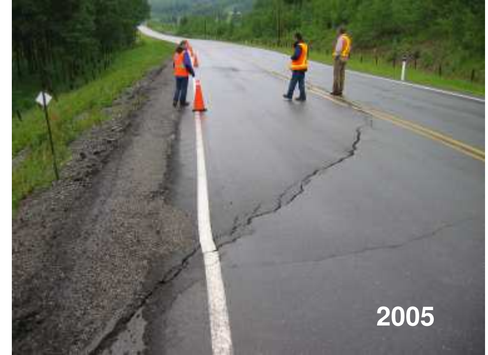
Photo S10(A)-2 – June 2005 (upper right) Settlement and cracking of the road surface as seen during the 2005 annual inspection. This pattern of damage to the road surface has been ongoing for the last several years, and was most recently noted during the borehole drilling and instrument installations in the spring of 2007 prior to the June 2007 inspection and photos.
