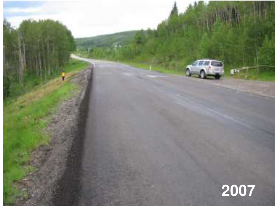
Photo S10(A)-1 – June 2007 (upper left) Facing north across the site. The recent overlay has obscured any recent cracking and settlement in the road surface. See Photo S10(A)-2 for a view of the site as it appeared during the 2005 inspection.
