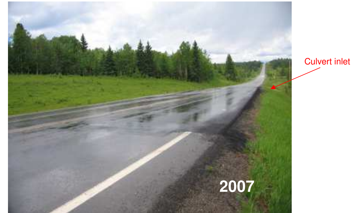
Photo S10(C)-2 – June 2007 (upper right) Typical view facing north across the recent overlay at the site, as seen during the June 2007 site inspection. The approximate location of the culvert to the south of the overlay is shown.
