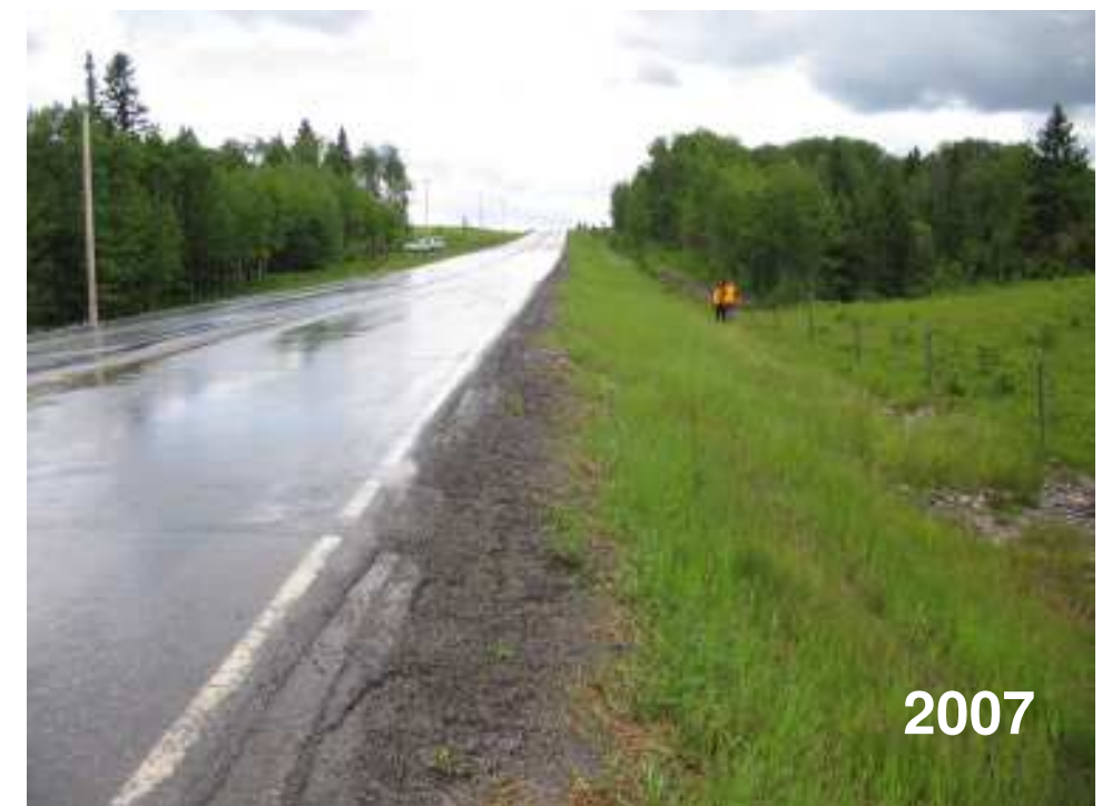
Photo S10(C)-4 – June 2007 (lower right) Facing south along the west shoulder of the road. The culvert shown in Photos S10(C)-5 and 6 is just behind the two people standing in the ditch to the right of the road.
