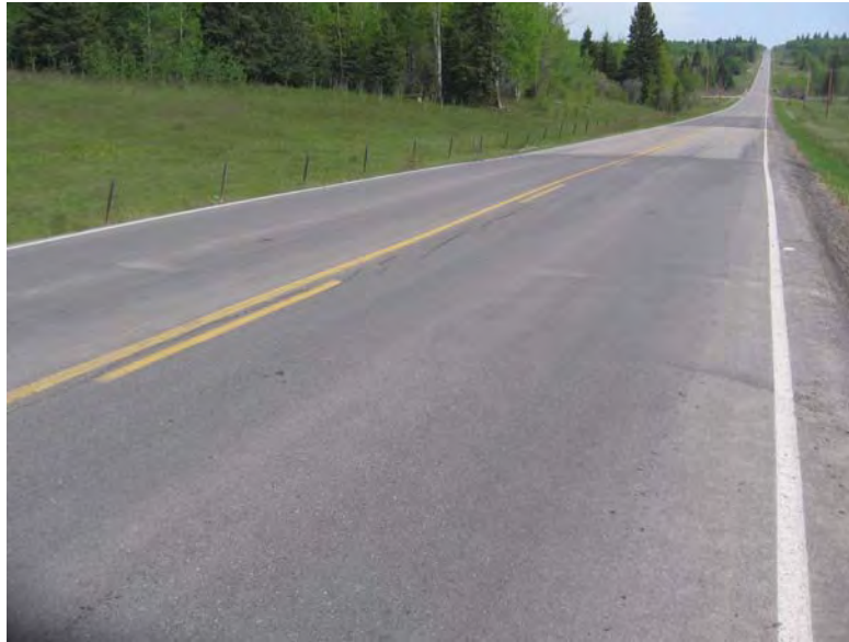
Photo S10(C)-3 (top) – June 2009 Facing northbound across the asphalt overlay to the north of the culvert. Cracking and settlement of the northbound lane has formed through repeated overlays since 2003.
