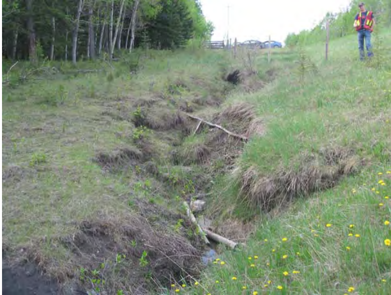
Photo S10(C)-5 (top) – June 2009 Facing southbound along the east road ditch, immediately south of the culvert outlet.
