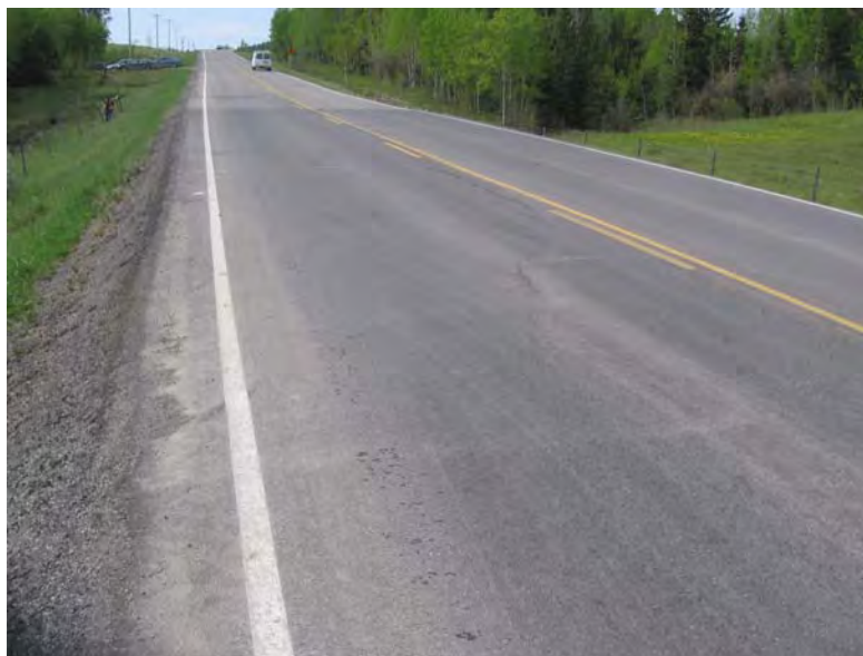
Photo S10(C)-4 (bottom) – June 2009 Facing southbound across the area shown in Photo S10(C) – 3. The minor cracking and settlement of the northbound lane that is visible in this photo has formed since the most recent overlay in 2008.
