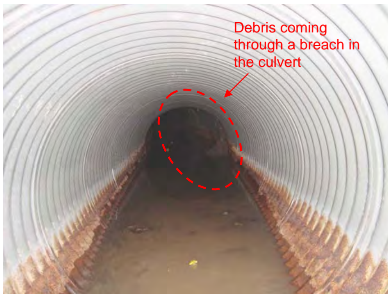
Photo S10(C)-2 (bottom) – June 2009 Facing downstream from the culvert inlet, with soil debris coming through a breach in the top of the culvert faintly visible in the right background.
