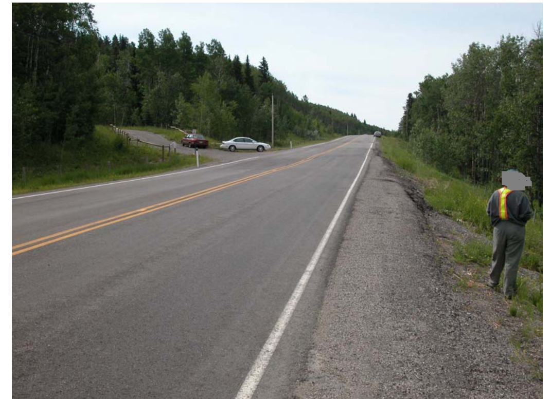
Photo 4 (lower right) Site A Facing south across Site A. The patched area with new cracking shown in Photo 1 is marked.
