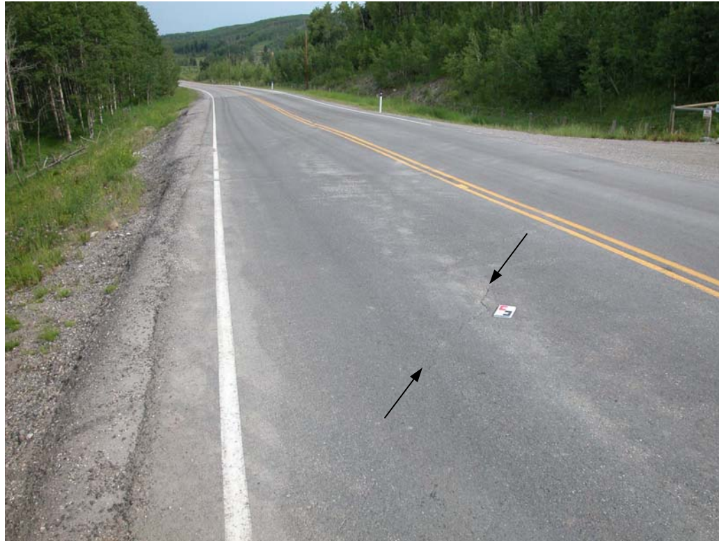
Photo 3 (lower left) Site A Another new crack forming at Site A (notebook on road surface for scale). The area shown by Photos 1 and 2 is visible in the background.
