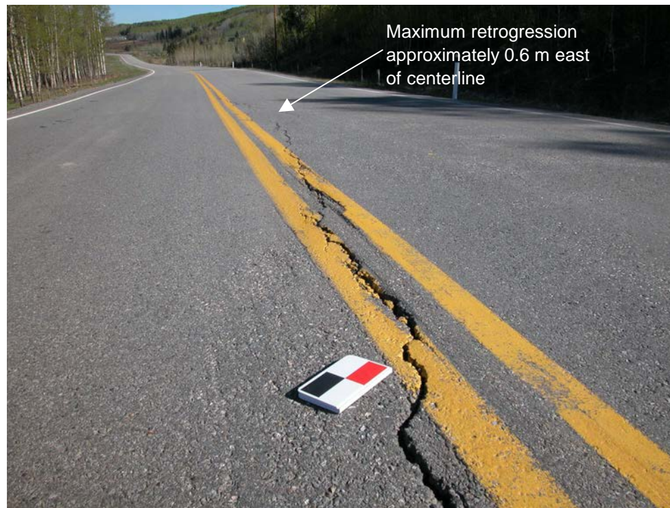
Photo S10A-5 (left) – May 2004 – close-up view (facing north) of the cracking along the centerline in the main cracking area. Lateral separation approximately 20 to 25 mm. Vertical displacement approximately 25 to 50 mm. It appears that the visible cracking and displacement has developed since the July 2003 inspection and subsequent repaving of the road through this area.
