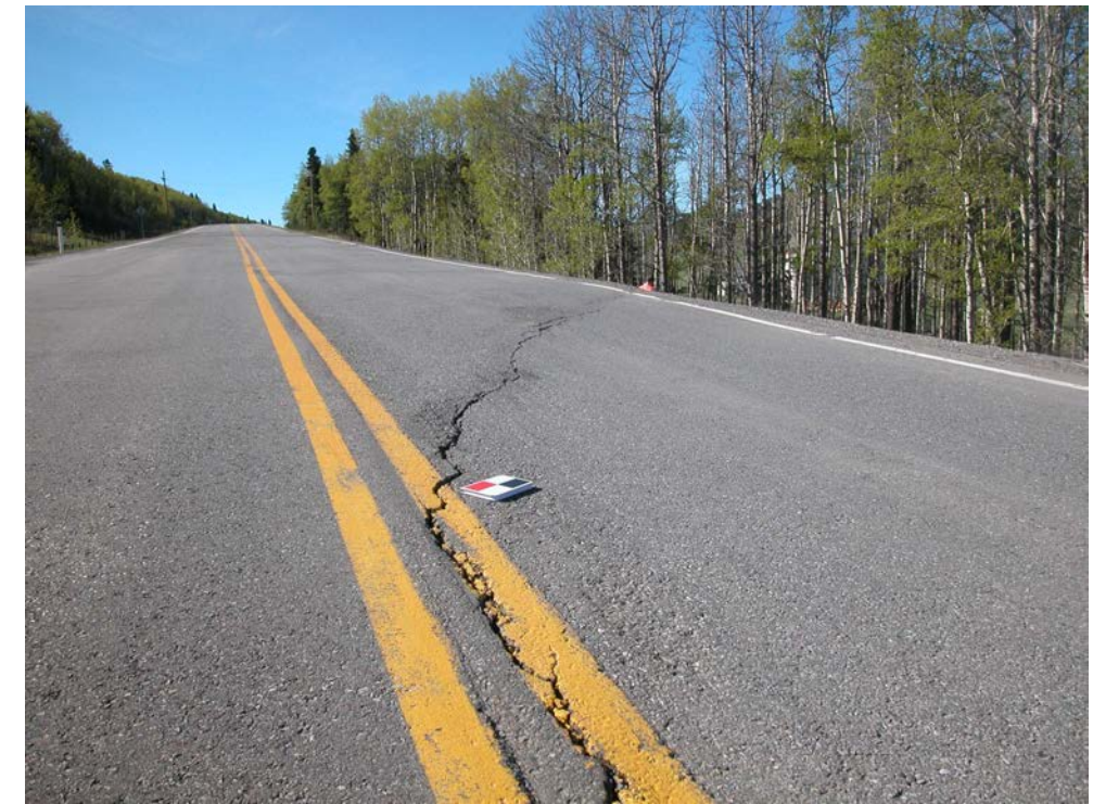
Photo S10A-6 (right) – May 2004 – close-up view (facing south) of cracking along centerline in main cracking area. Same area as shown in Photo S10A-5.
