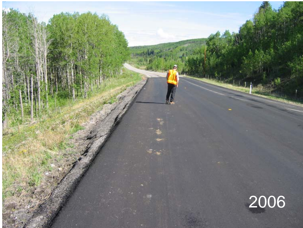
Photo S10(A)-1 (upper left) – May 2006 – facing north across the segment of the road where ongoing cracking and settlement has been noted since 2000. The area was repaved shortly before the time of the annual inspection, therefore it was not possible to check for further development of the previously noted cracking and settlement. Compare with Photos S10(A)-3 and S10(A)-4 which show the settlement and cracking in this area in June 2005.
