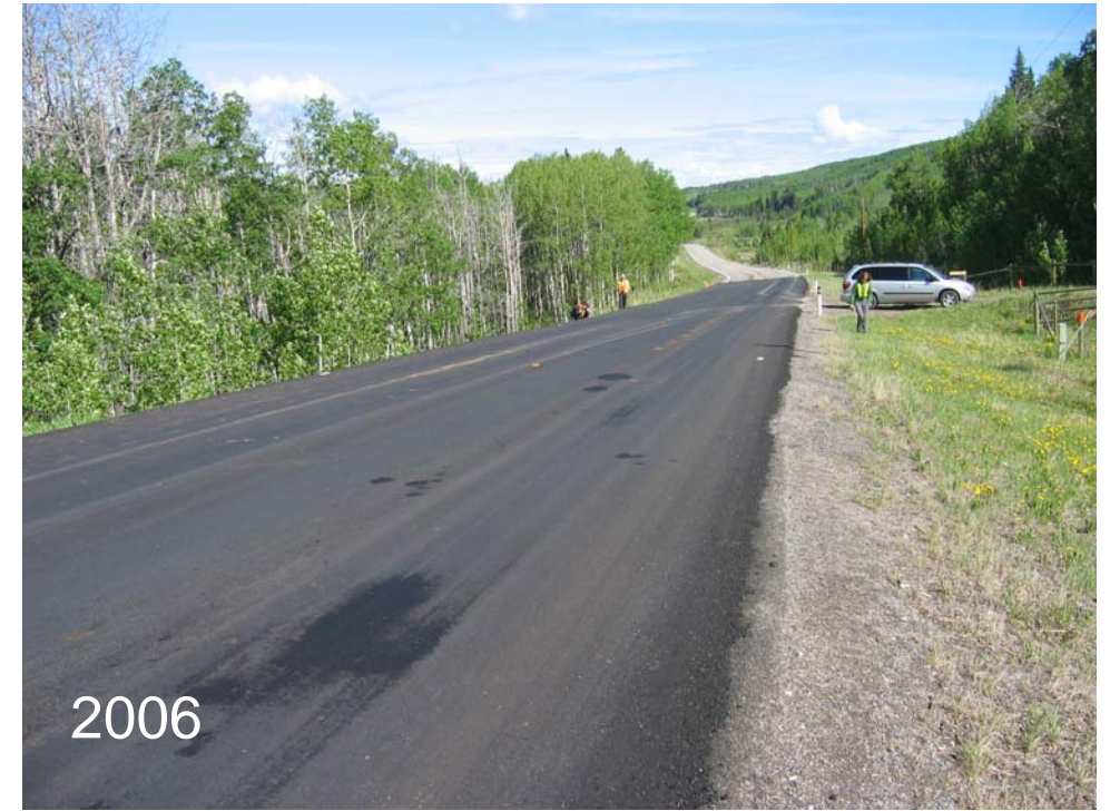
Photo S10(A)-2 (upper right) – May 2006 – another view of the previously-noted cracking and settlement area, facing north along the road. The area was repaved shortly before the time of the annual inspection. Compare with Photos S10(A)-3 which show the same area in June 2005.
