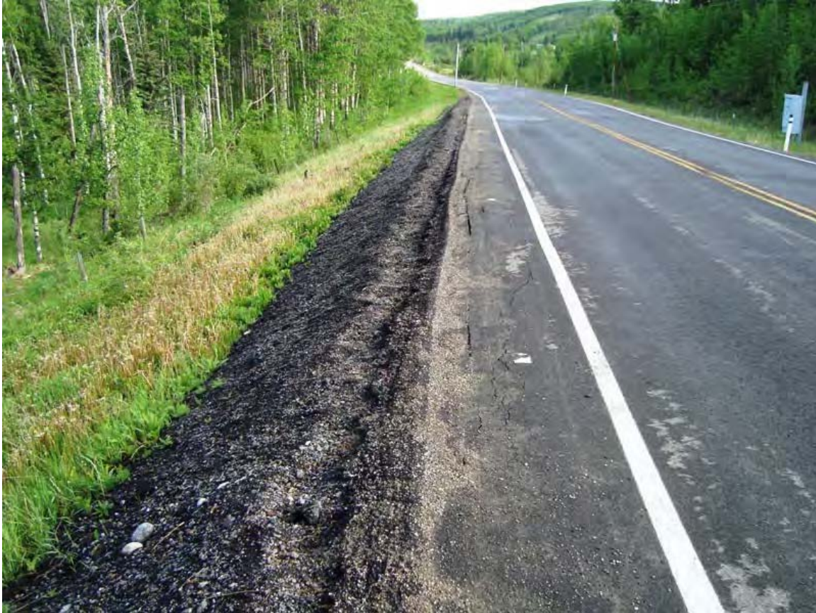
Photo S10A - 1 (June 2012) - Facing north from the south end of the site. An overlay was placed at the site in late 2011. Subtle cracking and settlement had formed through the overlay following similar extent as was observed in 2011 and in previous inspections.
