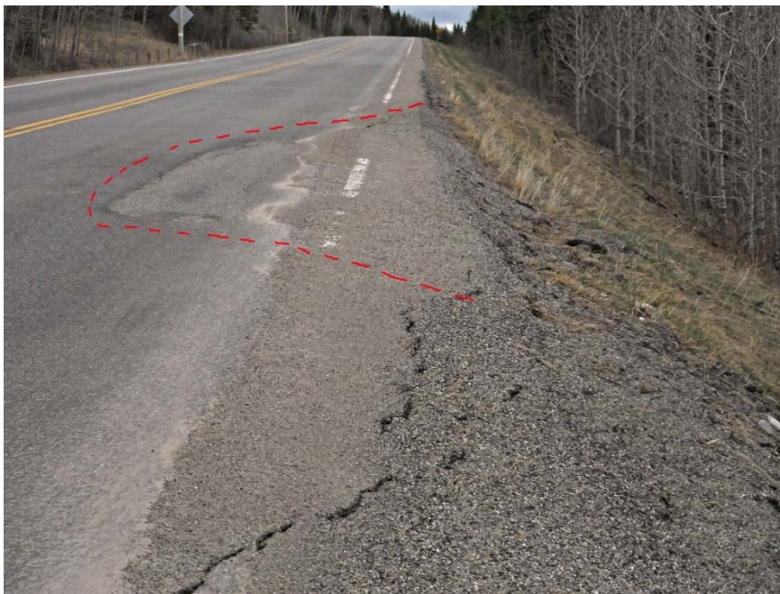
Photo S10A - 2 (May 2014) - Facing south at the new damage observed in the road surface, at the south end of the main slide area seen in the previous photo. The approximate extents of the newly observed damage is outlined in red.
