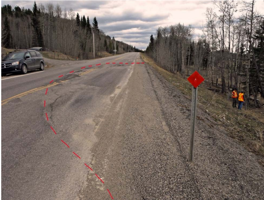
Photo S10A - 1 (May 2014) - Facing south from the north end of the site. Cracking and settlement had formed through the previous overlay following similar extent as was observed in 2012 and in previous inspections. The approximate extents of the main slide area within the road is outlined in red.
