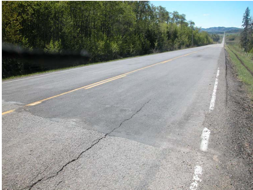
Photo S10B-1 (upper left) – May 2004 – facing south across the July 2003 overlay at Site B. There is longitudinal cracking visible at the north end of the overlay (foreground of photo) but judged to be a pavement phenomenon rather than indicating geotechnical instability.
