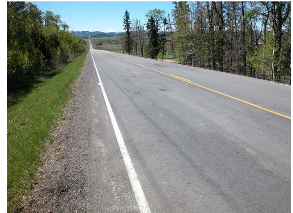
Photo S10B-4 (lower right) – May 2004 – general view facing south across the July 2003 overlay at Site B.
