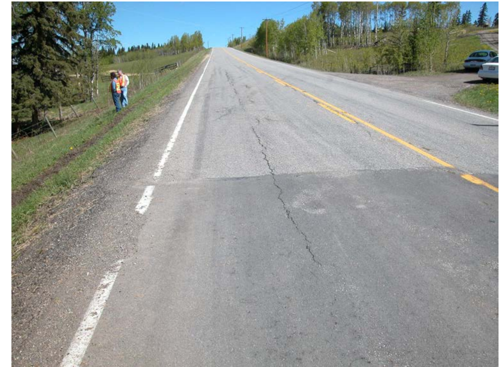
Photo S10B-2 (upper right) – May 2004 – facing north. Another view of the longitudinal cracking at the north end of the July 2003 overlay at Site B.
