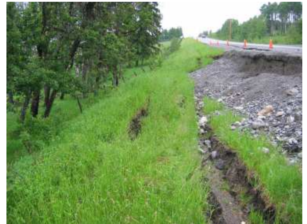
Photo S10(B)-4 (upper left) – June 2005 – deformation of slope face to west of road and tilted trees indicate that the overall toe of the failure extends to the west of the fence line.
