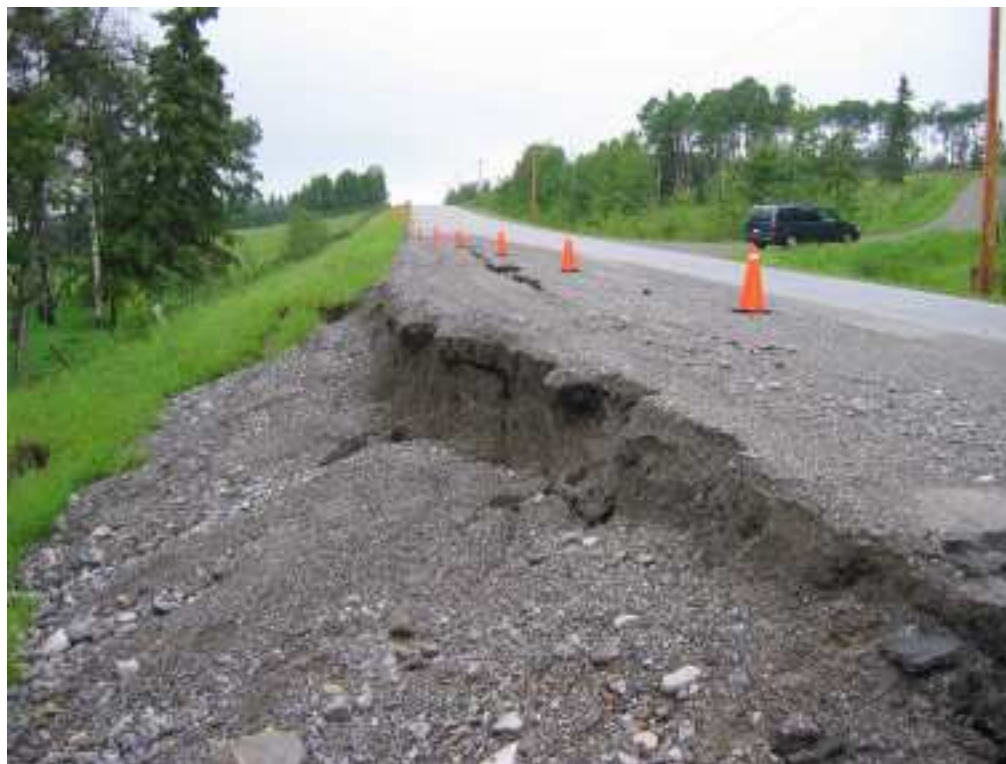
Photo S10(B)-3 (lower left) – June 2005 – closer view of north flank of the main failure area.
